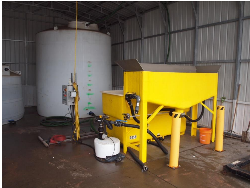
Figure 22 – AccuBatch Brine Maker located at the NTEMP S3 maintenance facility (Source: photograph taken on April 29, 2021, by NTSB investigators).
