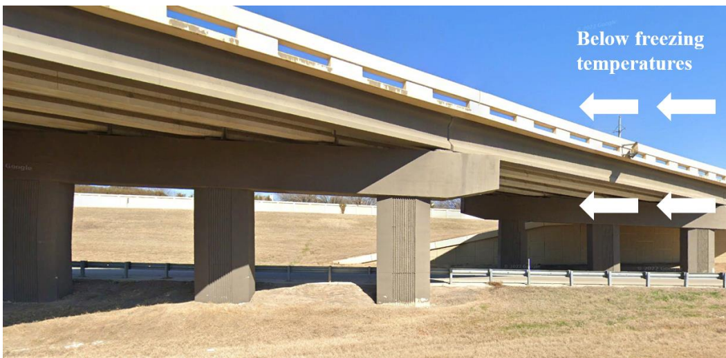
Figure 24 – Underside of a generic bridge. White arrows represent surrounding air on all sides of the bridge and not wind direction (Source: Google Earth Street view image revised).
