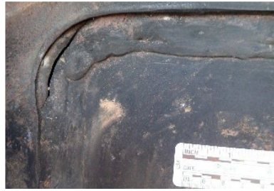
17(b). Cracked A-end A-3 weld, left forward corner.
