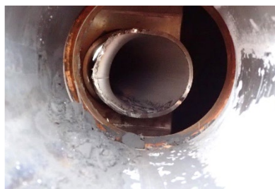
Figure 20. Flared (impact damaged) eduction pipe bottom as seen through the open bottom outlet ball valve, TILX 731748. January 27, 2022.
