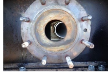
19(c). Displaced eduction pipe and flange as seen through BOV hole (investigators removed the bottom outlet valve from the flange).
