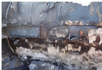
13(d). No breaching damage identified at the B-end stub sill inboard at tail piece following jacket removal.
