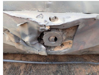
Figure 12. BOV stem adapter with top surface torsional fracture. Slotted end was severed and missing, CRDX 300073. January 27, 2022
