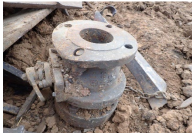
8(b). Separated 3-inch top valve with impact damage.
