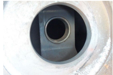
8(c). Eduction pipe flange over BOV opening.
