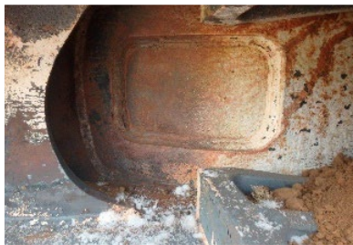
16(d). A-3 window weld, viewing the interior surface of the stub sill top plate.
