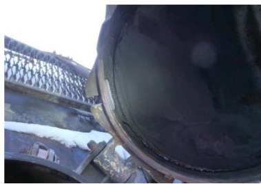
4(b). Thermally destroyed manway gasket and carbon on interior of manway cover.
