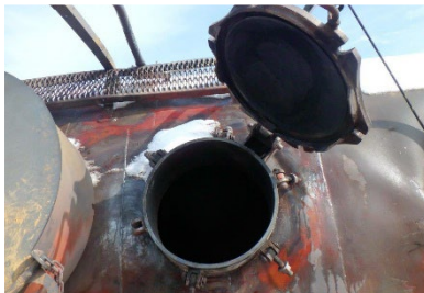
9(a). Thermal damage to tank jacket around the manway.
