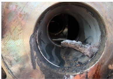
13(a). Mass of melted and extruded Teflon ball valve packing and eduction pipe flange seen through the BOV hole.
