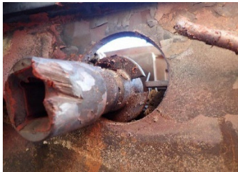
Figure 10. BOV stem adapter with witness mark/ contact damage without breakage at shear groove, CRDX 300133. January 11, 2022. Courtesy Trinity Industries Leasing, Inc.
