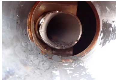
7(d). Flared (impact damaged) education pipe bottom as seen through the open bottom outlet ball valve.
