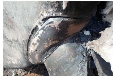
7(c). Fractured A-1 and A-2 head pad welds and cracked head brace-to-head pad weld.
