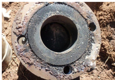
10(d). Thermally damaged liquid valve gasket.
