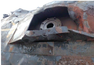
8(a). Collapsed portion of skid protection structure with bottom outlet valve missing.
