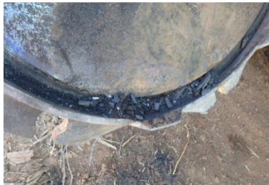
8(d). Thermally damaged manway gasket material.
