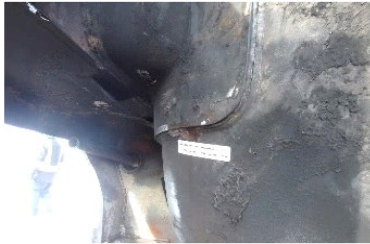
19(a). B-end head pad with cracked A-1 and A-2 fillet welds.
