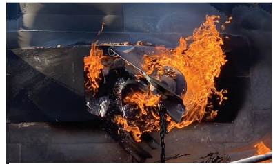
15(c). BOV active leak with fire due to burned out seats and gaskets.
