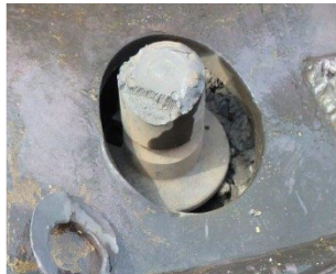
Figure 11. BOV skid protection structure, shallow dent A-end side (right side in photo). BOV handle adapter not sheared and BOV ball valve seen partially open, CRDX 300073. January 27, 2022
