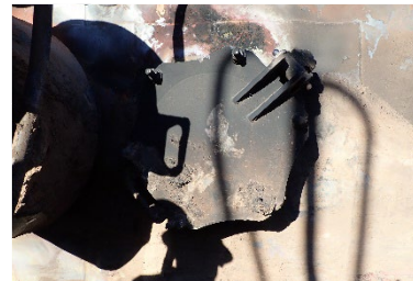
2(c) Thermal damage to manway with visible carbon on lid.
