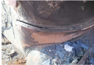
7(b). Fractured A-2 head pad weld and separated head pad.
