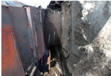
3(a) A-end head pad and head brace. No breach.
