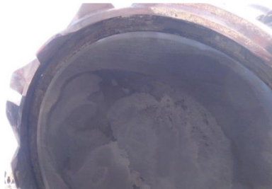
9(b). Internal surface of manway cover with thermally damaged gasket.
