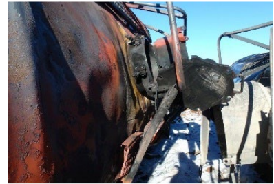
18(c). Scorched jacket surrounding manway and top fittings housing. Thermally damaged gasket material was hanging loose from the open manway.
