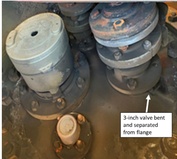
Figure 15. Three-inch valve sheared from flange below damage to protective housing. CRDX 300133. Courtesy Federal Railroad Administration, January 11, 2022.
