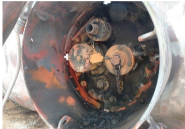
3(b) Thermally damaged top fittings.
