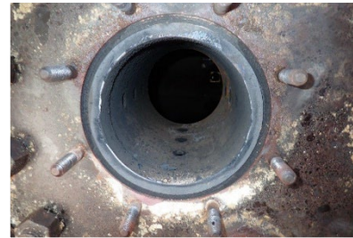
10(c). Carbon deposits on internal surface of PRD vapor space communication pipe.
