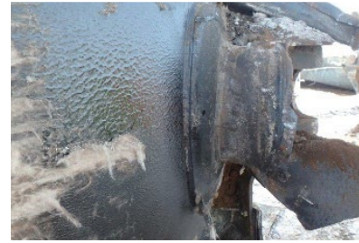
17(c). A-end head pad and head brace. The head pad A-1 and A-2 welds were not fractured.
