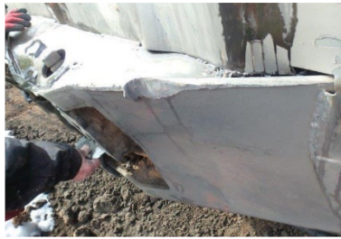
11(b). Skid protection structure impact mark, A-R side of skid structure.
