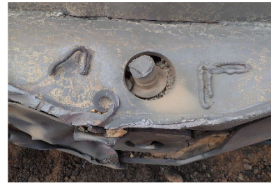
11(c). BOV stem adaptor with top surface torsional fracture. Slotted end was severed and missing.
