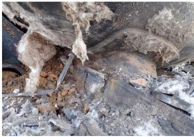
14(b). Fractured stub sill web at head brace and head pad. No tank breaching damage in this area.
