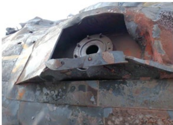
Figure 5. Center skid structure collapsed, shearing full BOV assembly and ball valve, TILX 731739. January 27, 2022.
