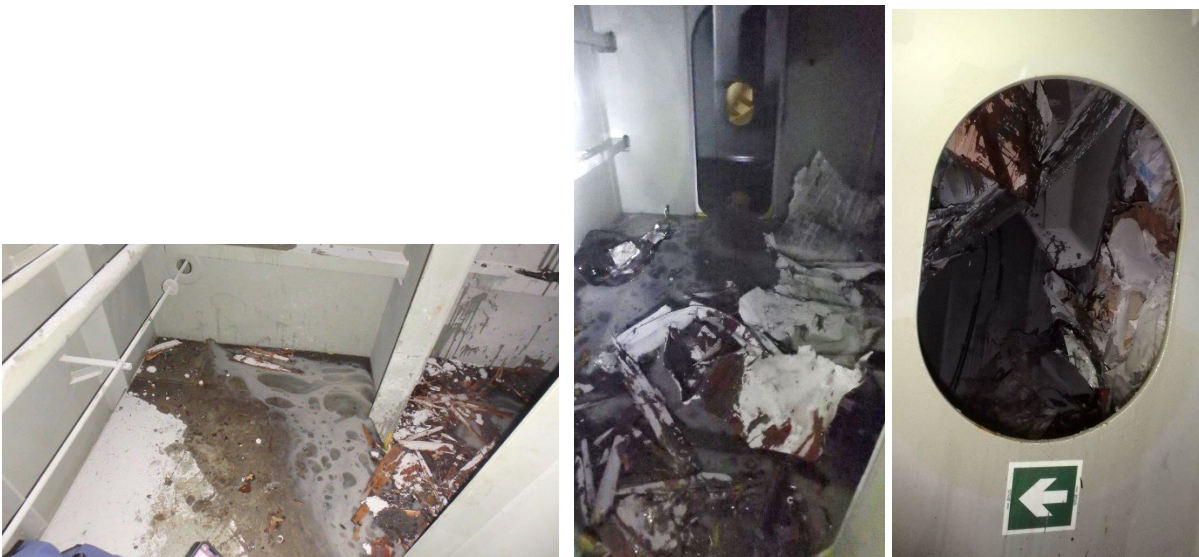
Figure 24. 2 nd Deck below Bays 6-10. Surfactant-like material on deck at bulkhead between Bays 6 and 10 (left); view into area below Bay 6 with fallen debris and accumulating liquid (center); view through bulkhead into area below Bay 6 with liquid dripping from above (right). March 28, 2024.
