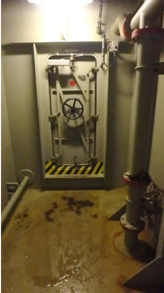
Figure 25. Viscous non-volatile sticky liquid leaking from the Bay 2 bow thruster room water-tight door. March 28, 2024.
