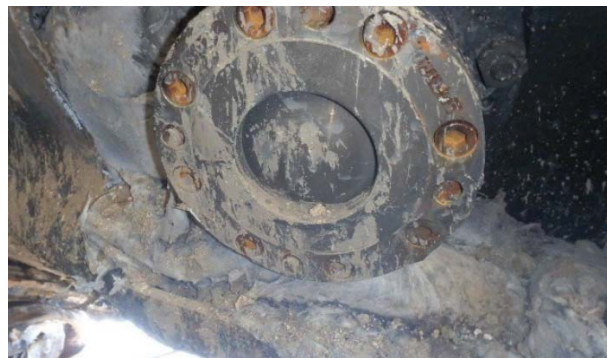
6(d) Thermally damaged BOV with missing nozzle.
