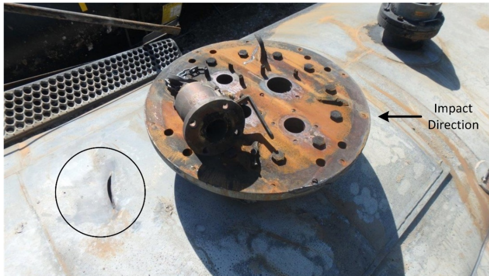
Figure 5. Top fittings flange showing missing multihousing cover, vapor valve, liquid valve, and VRV. A dent and jacket tear occurred on the opposite side of the flange (circled).
