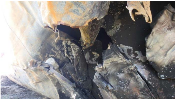
5(c) Fractured tank shell in B-R bolster region.
