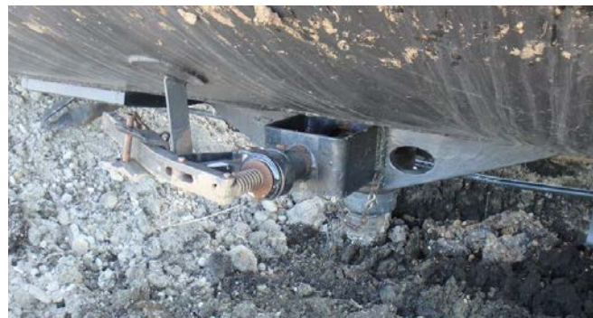
14(d) BOV operating handle and undamaged nozzle extension.
