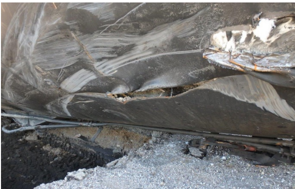
12(c) B-L longitudinal jacket tear below shell gouge.
