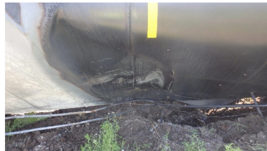
9(b) Buckled A-L shell and thermal damage to jacket.
