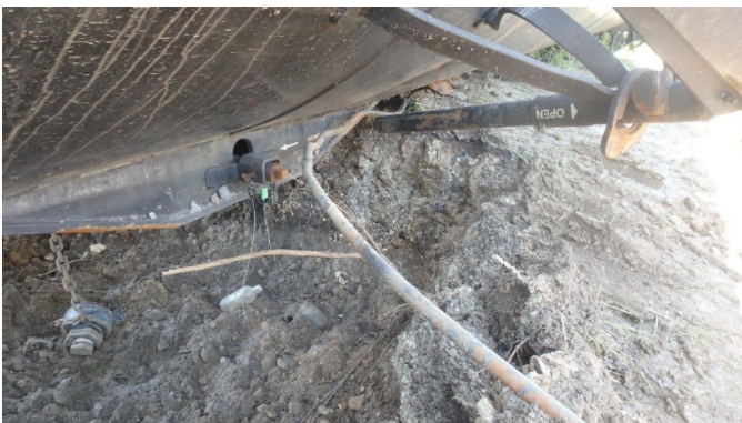
11(c) BOV operating handle separated from the ball valve extension shaft.
