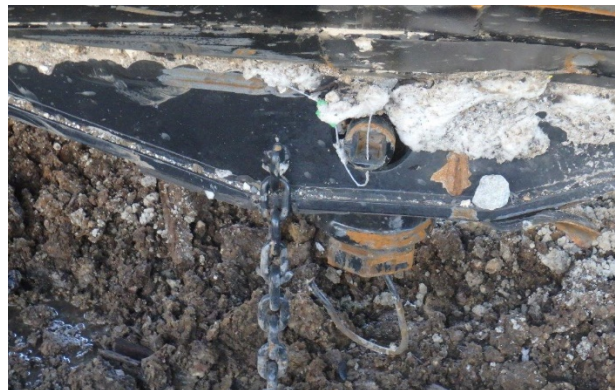
3(d) BOV missing operating handle and undamaged nozzle.
