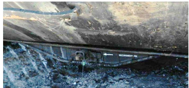
15(d) Missing BOV operating handle and undamaged nozzle extension. The ball valve extension shaft securement pin was in place.
