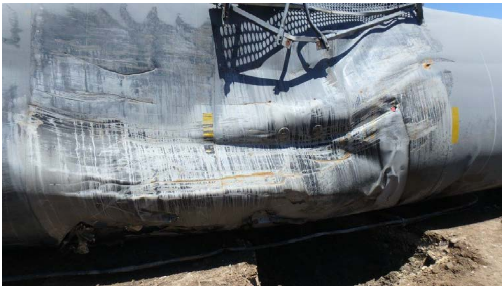
Figure 8. Dent and jacket damage to left of tank puncture.
