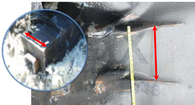
8(c) Stub sill 14” impact mark in A-L shell. The tank jacket is still in place. Inset photo is the stub sill of TILX 351873 showing relationship of impact mark to contact surface.
