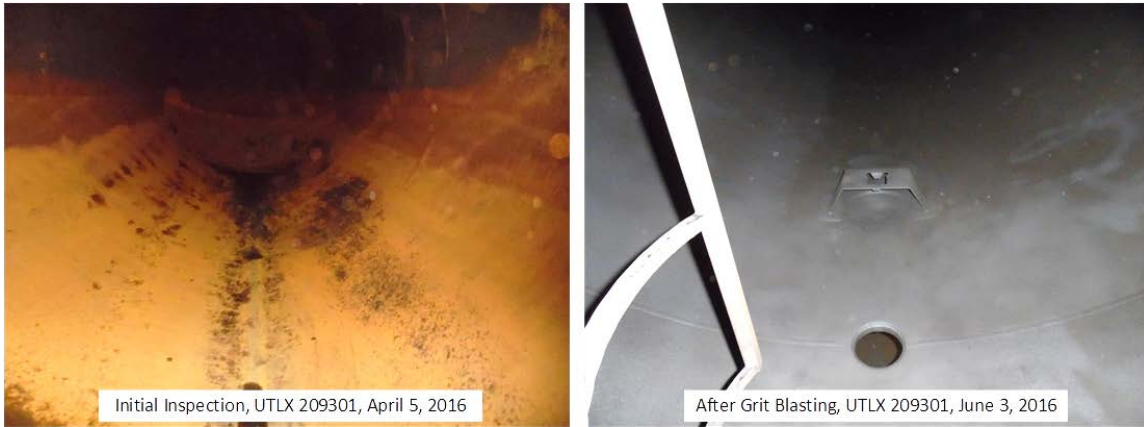
Figure 11. Before and after grit blasting. Views of the interior surface of UTLX 209301 during the 2016 shopping for qualification inspection, courtesy of Union Tank Car Company.
