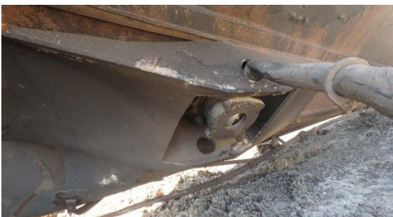
7(g) Open BOV ball valve, bent operating handle and fractured skid weld.
