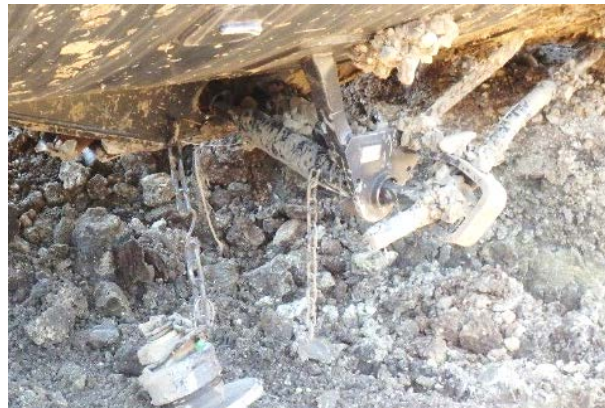
17(d) The BOV operating handle was bent, with extension sleeve disengaged from the valve stem.
