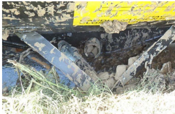
13(d) The BOV operating handle sleeve bent away from ball valve extension.
