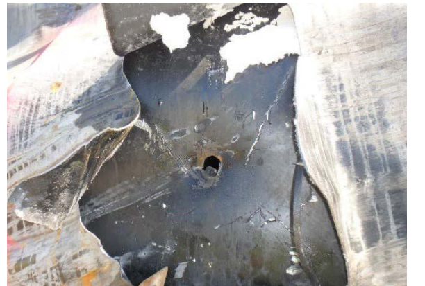
16(d) Tank jacket peeled away from the puncture location.
