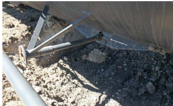
18(d) BOV operating handle and nozzle were missing, securement pin was in place.
