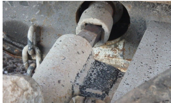
2(d) Bent BOV operating handle shaft and extension.
