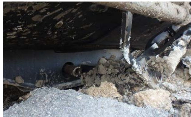
12(d) The BOV operating handle sleeve was bent away from the ball valve extension.
