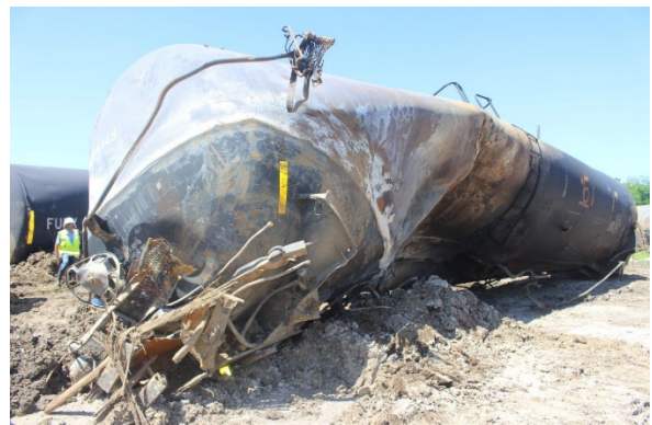
7(f) Buckled B-R side and thermal damage.
