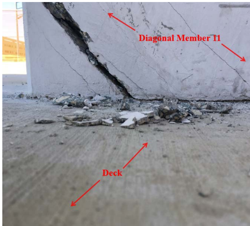
Figure 4. Location: Bottom of diagonal member 11 east face, looking to the west. Time stamp: March 13, 2018, at 1:29:15 p.m., labels added by the NTSB. (Source: Munilla Construction Management)
