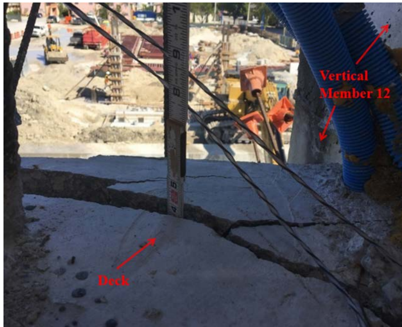
Figure 1. Location: Diaphragm II, west side directly adjacent to vertical member 12, top deck view of crack, looking to the north. Time stamp: March 13, 2018, at 11:16:50 a.m., labels added by the NTSB. (Source: Munilla Construction Management)
