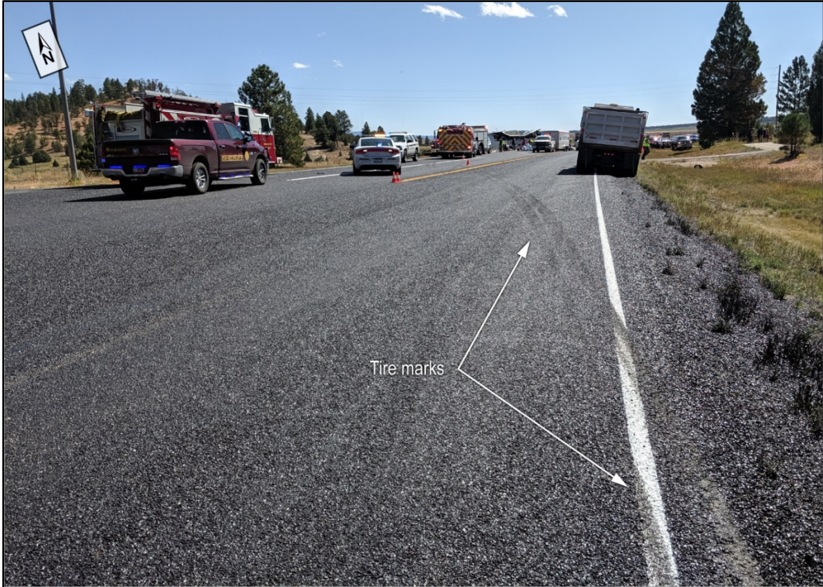
Figure 4. Tire marks curving across eastbound travel lane after bus departed roadway and was steered back. (Source: Utah Highway Patrol)
