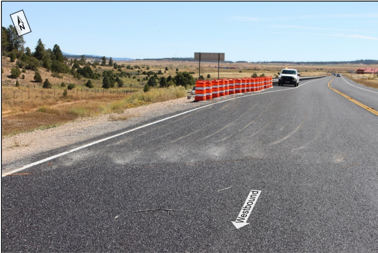
Figure 6. Gouge marks on westbound lane pavement left by bus sliding toward guardrail.
