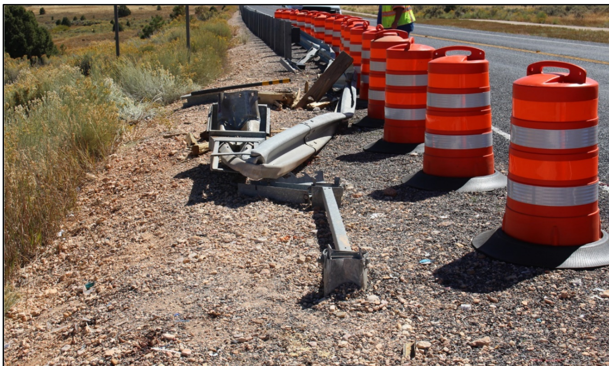
Figure 7. Damaged guardrail on westbound side of SR-12. (View is looking east.)
