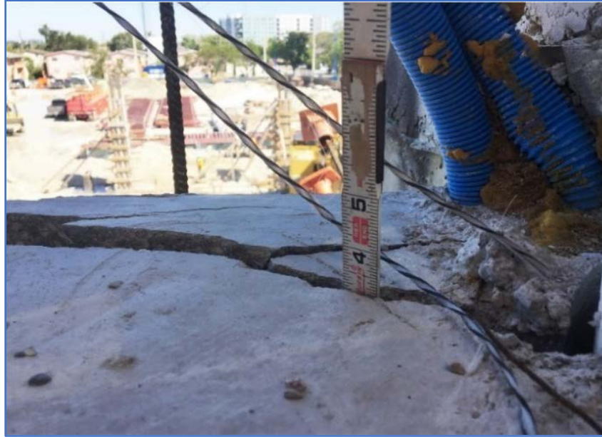
Figure 24. Cracks of 3–4 inch depth at northern end of precast main span, along west side of diaphragm 2 (north view), March 13, 11:17 a.m. (Source: MCM)
