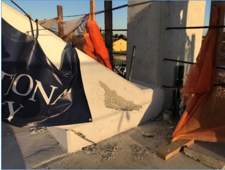
Figure 26. Cracks at bottom of diagonal member 11 (east view), March 15. (Source: FIGG)
