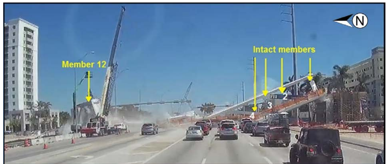
Figure 11. Still image (time stamp 13:46:44:310) from in-vehicle mounted video camera on pickup truck traveling east on SW 8th Street, showing main span completely collapsed, March 15, about 1:46 p.m.
