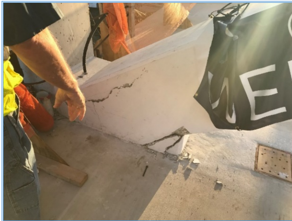
Figure 25. Cracks at bottom of diagonal member 11 (west view), March 15. (Source: FIGG)
