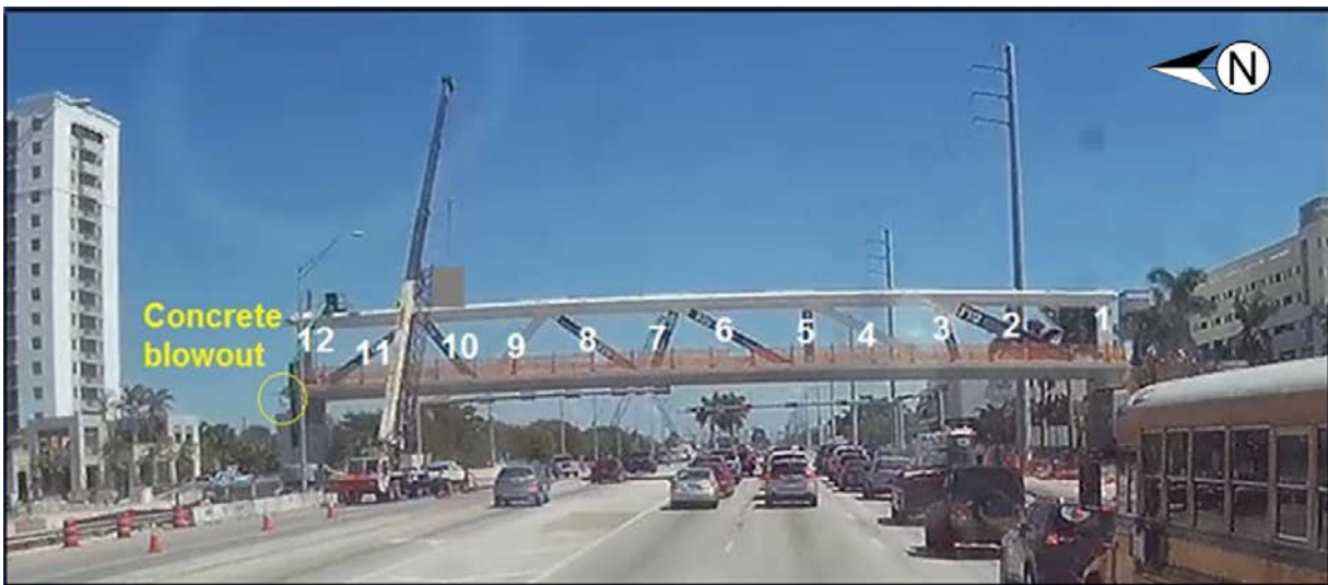
Figure 9. Still image (time stamp 13:46:43:881) from in-vehicle mounted video camera on pickup truck traveling east on SW 8th Street, showing concrete dust and debris blowout at north end (pylon pier), March 15, about 1:46 p.m.
