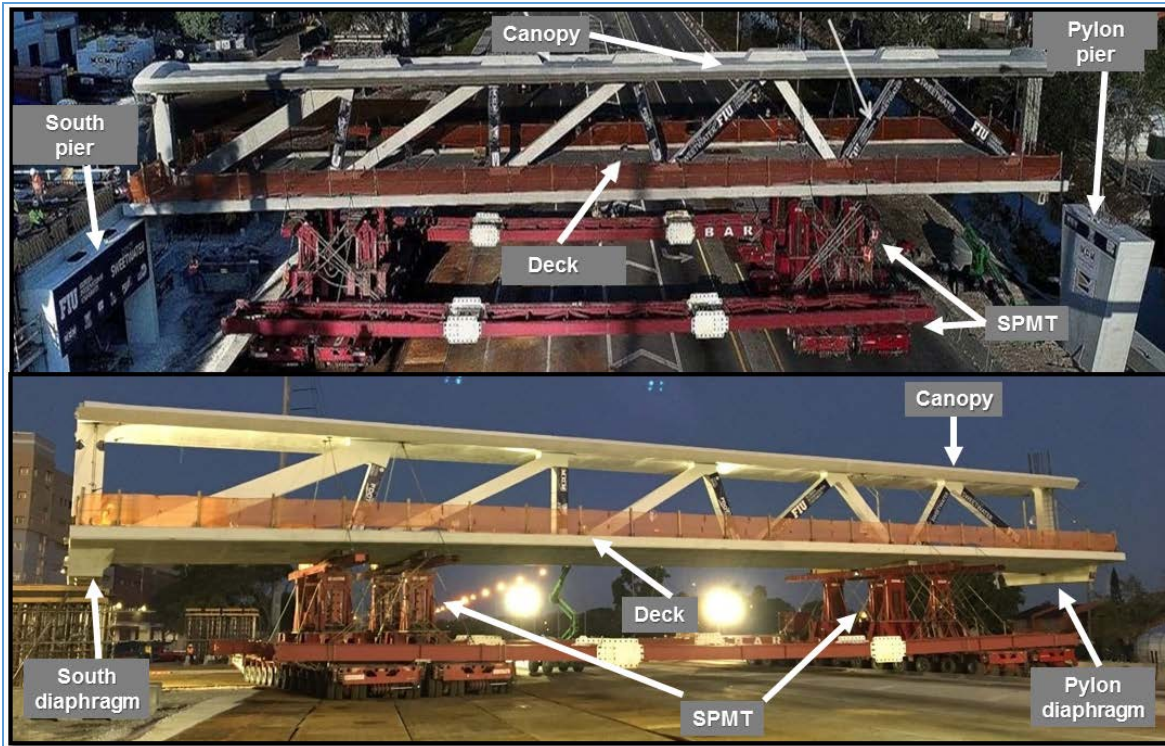
Figure 22. SPMT being moved overnight on March 10 (bottom) and main span being placed on south and pylon piers, facing west (top). Transport occurred over 8 hours, starting at 4:30 a.m., with placement of final permanent pier support concluding at 12:30 p.m. (Source: FIGG, annotated by NTSB)
