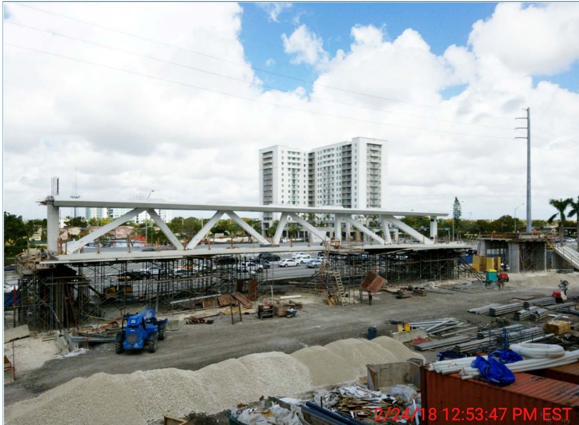
Figure 15. Temporary falsework supporting the bridge span in the casting yard on February 24, 2018, being sequentially removed from the middle of the span toward the ends of the span. (Source: MCM)
