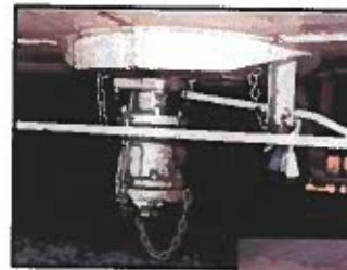
Internal Bottom Outlet Valves
