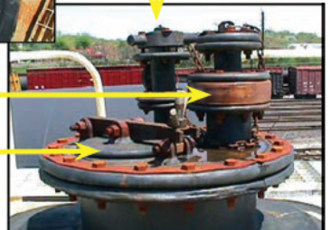
Safety Vent/Air Line
