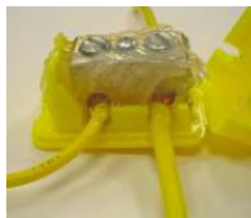
New Service Line to Plastic Main Connection
