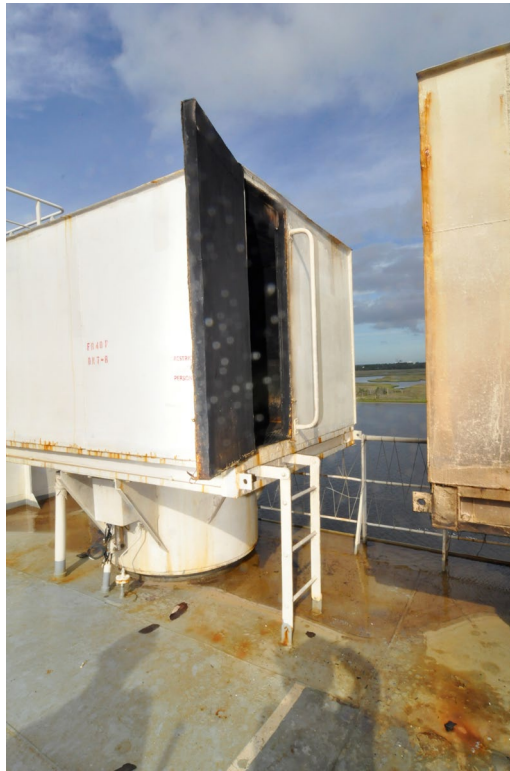
Figure 8. Vent 7S on the port side exhibiting soot on the interior of the open door.
