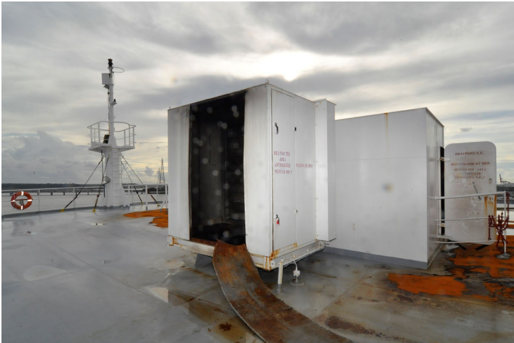
Figure 14. Vent 9E on the port side of the bow exhibiting soot staining near the top and mechanical damage consistent with overpressure on the outboard side.
