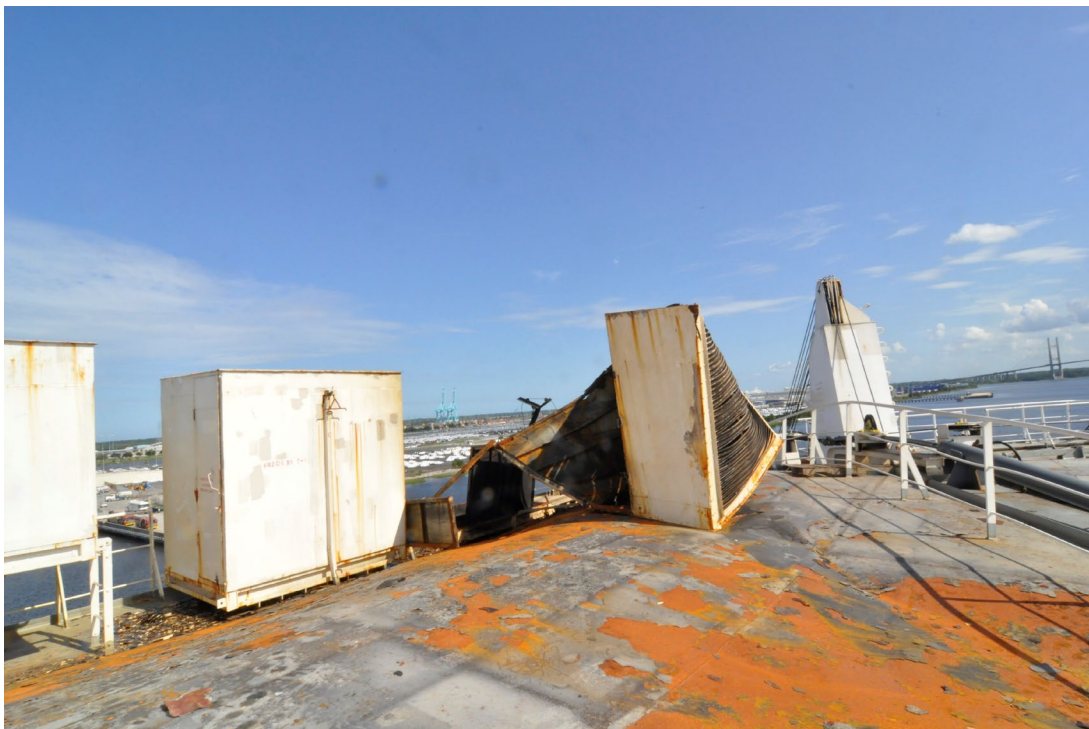
Figure 15. Vents 10E and 7E on the starboard side of the stern. Vent 10E exhibits mechanical damage due to overpressure. Vent 7E exhibits light soot staining on the upper corner.
