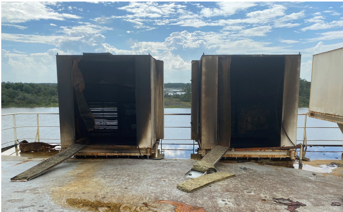
Figure 7. Vents 10E and 9E on the port side of the stern. Both exhibit soot staining and damage due to overpressure.
