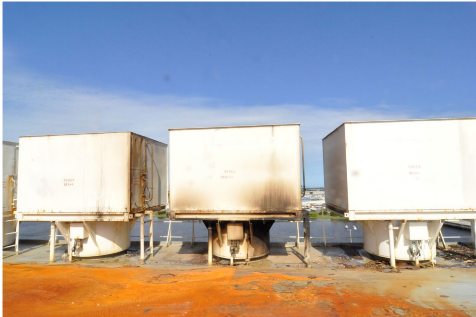
Figure 18. Vent 10S on the starboard side exhibiting soot staining on the exterior.
