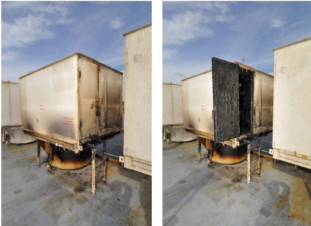
Figure 10. Two photos of vent 10S on the port side. Left: Exhibiting soot and thermal discoloration on the exterior. Right: Internal soot and thermal damage.
