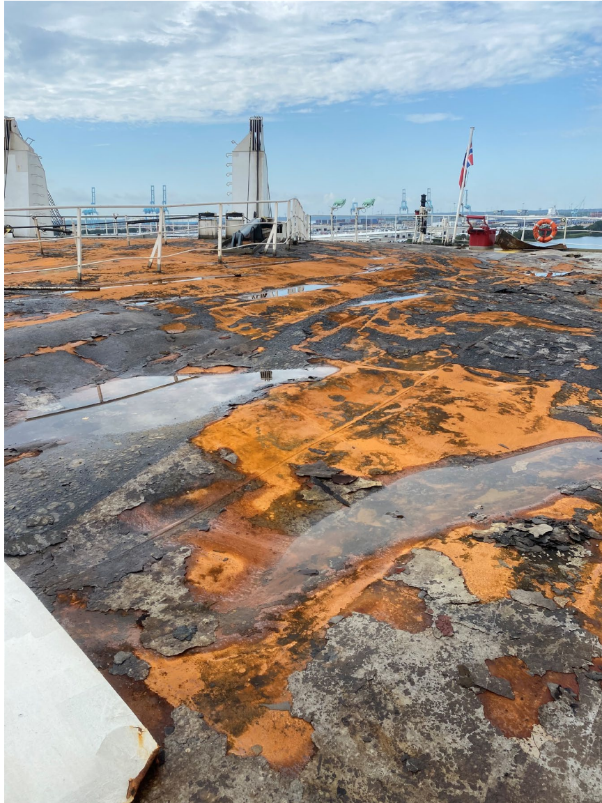
Figure 37. View from the port side toward the stern ramp. The surface of deck 12 is exhibiting deformation and charring/loss of paint.
