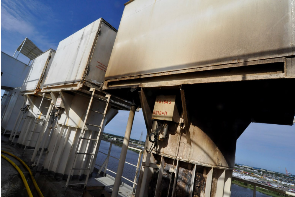
Figure 20. Vent 10S on the starboard side exhibiting soot staining on the exterior.
