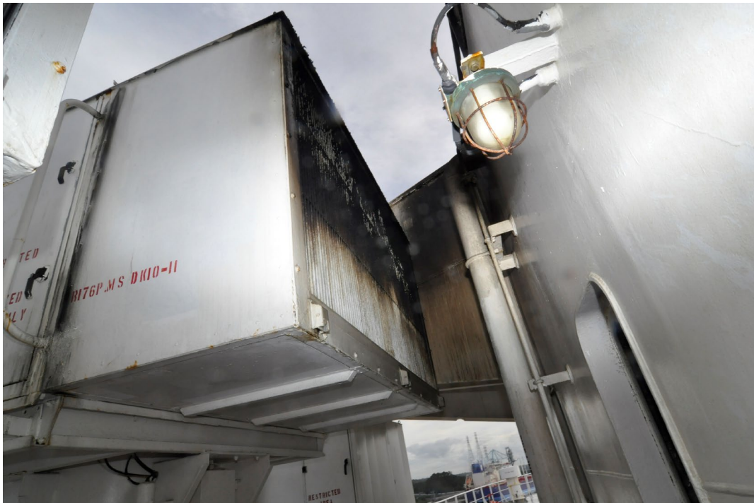
Figure 13. Vent 10S on the port side exhibiting heavy soot staining on the exterior.
