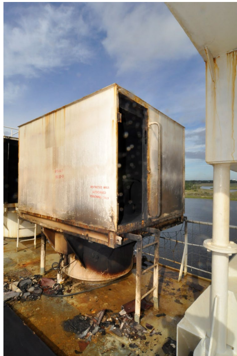
Figure 9. Vent 10S on the port side exhibiting soot and thermal discoloration. The doghouse door is missing, and there is debris around the base.
