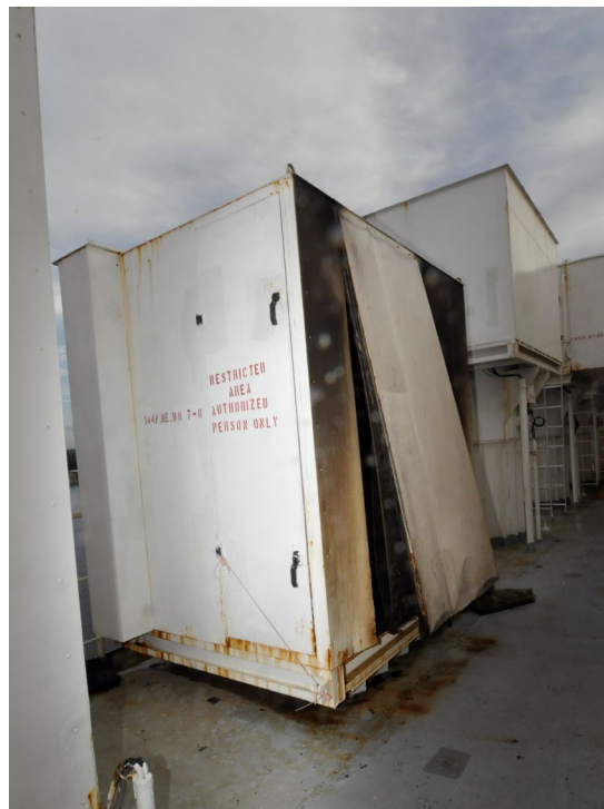
Figure 11. Vent 7E on the port side exhibiting external soot staining and the inboard doghouse wall displaced outward from the bottom.
