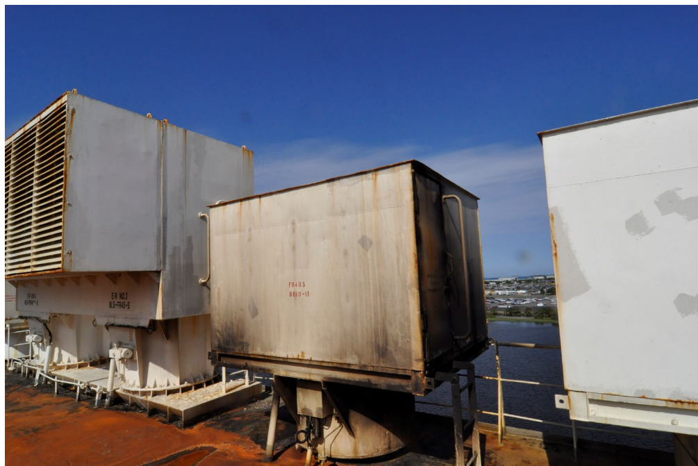
Figure 17. Vent 10E on the starboard side exhibiting external soot staining.
