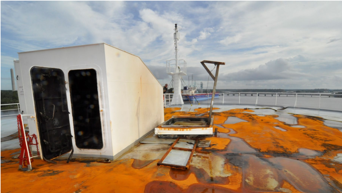
Figure 21. Vent 10E on the starboard side of the bow. The upper portion of the doghouse is completely separated from the base and missing. This mechanical damage is consistent with an overpressure event. There is soot staining on the bulkhead adjacent to where the doghouse had been.
