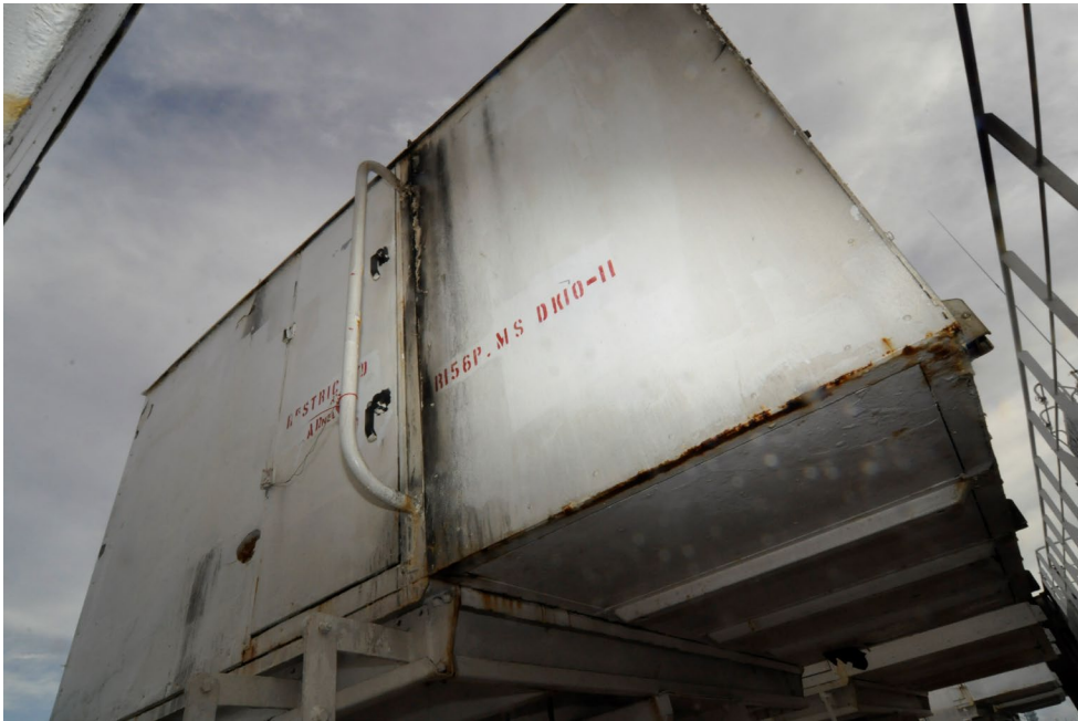
Figure 12. Vent 10S on the port side exhibiting soot staining on the exterior door seam.
