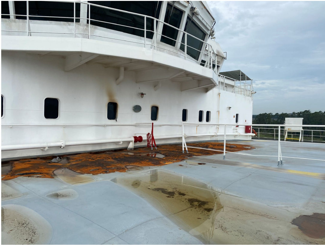
Figure 41. View of the area below the bridge, including thermal damage to the deck surface and smoke stains above the window of the space below the bridge.
