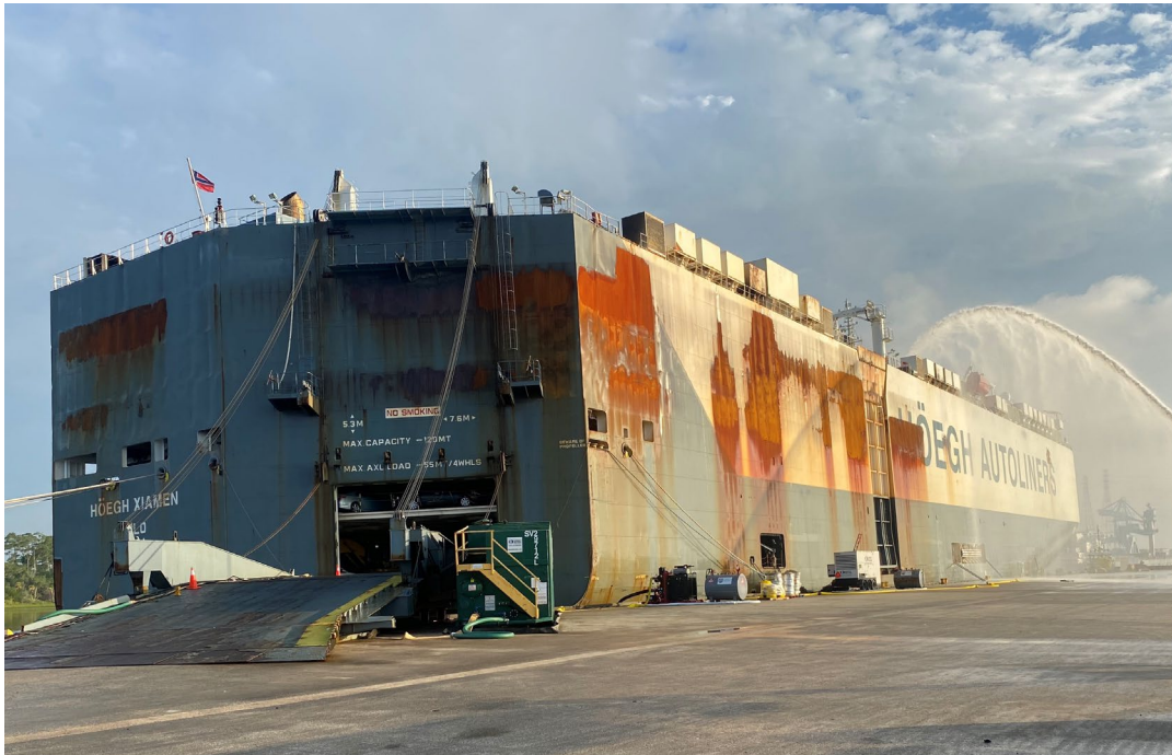
Figure 36. Thermal damage on the exterior skin of the ship denoting areas where the fire had been in proximity to the skin.
