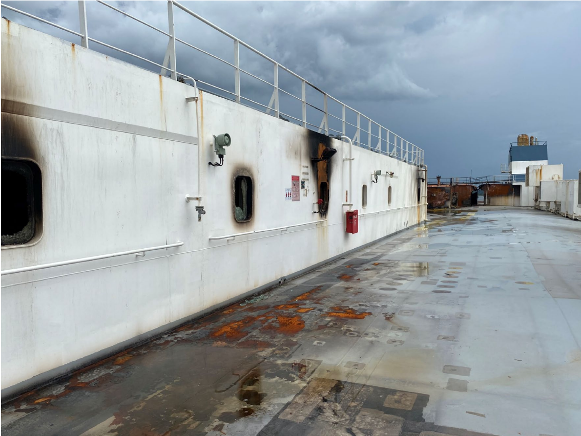
Figure 43. Thermal damage on the deck and smoke and thermal damage above the windows of the accommodation space on the port side.
