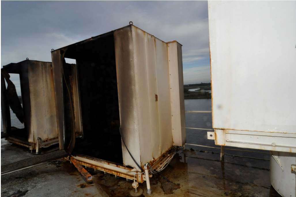
Figure 6. Vents 10E and 9E on the port side of the stern. Both exhibit soot staining and damage due to overpressure.
