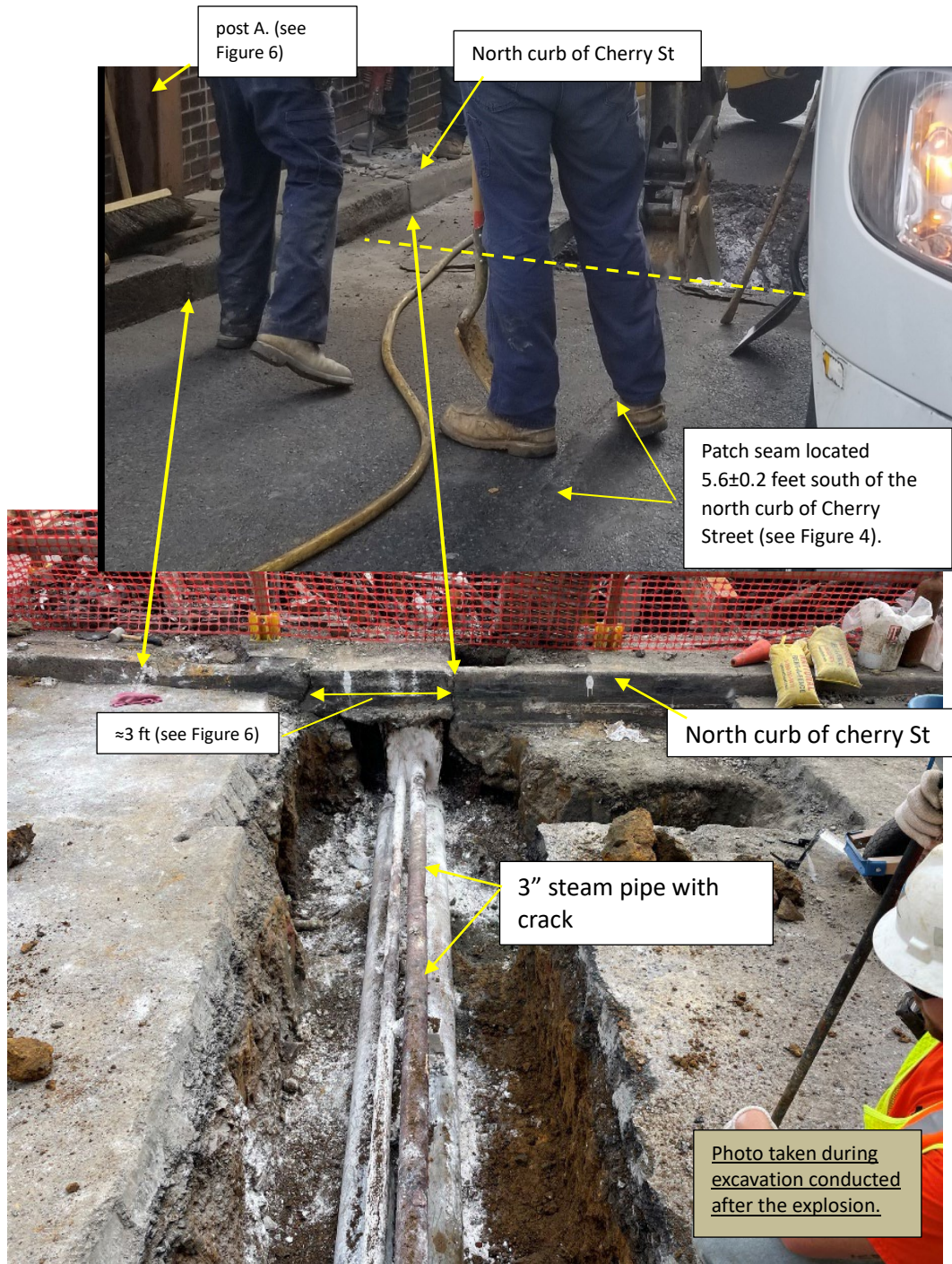
Figure 9. The upper image shows the work crew and excavation in the photograph taken on February 16, 2021 (Figure 2, zoomed). The bottom image was taken during the excavation conducted after the explosion. The broken yellow line shows the alignment of the west edge of the excavation with the north curb of Cherry Street. As indicated by the diagram the south edge of the excavation (hidden behind the truck) is located south of the pavement seam which is located 5.6 \pm 0.2 ft south of the north curb of Cherry Street (see also figures 3, 4 and 7).
