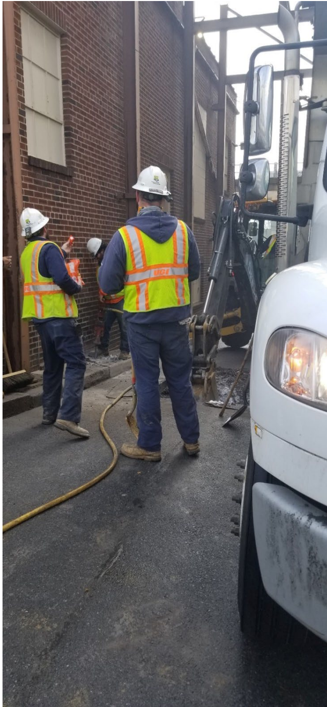
Figure 2. UGI Crew working on Cherry Street outside the Palmer Candy Factory on February 16, 2021. (Source: Palmer)
