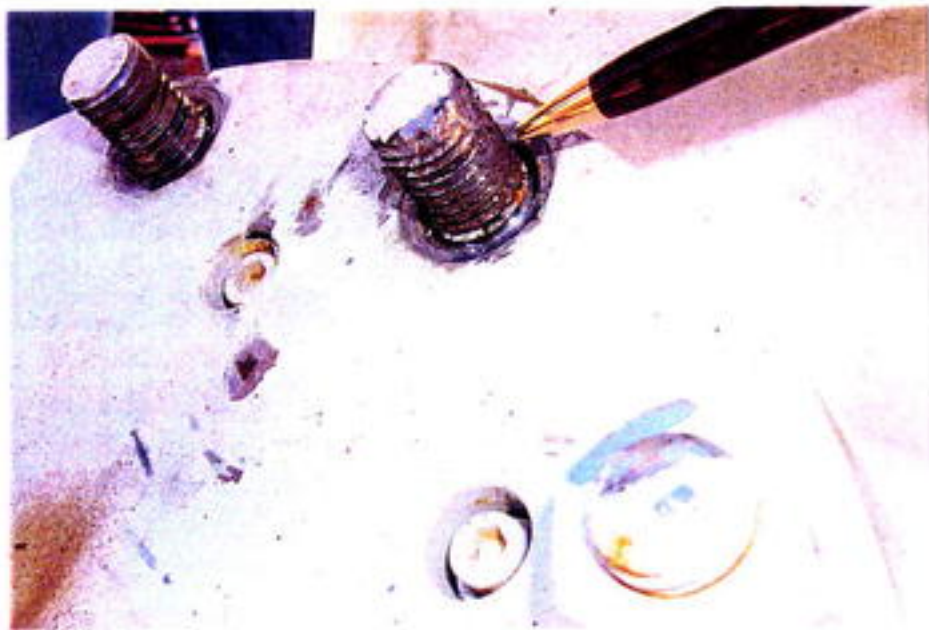
Figure 2.11 Missing Nuts and Damaged Stud
