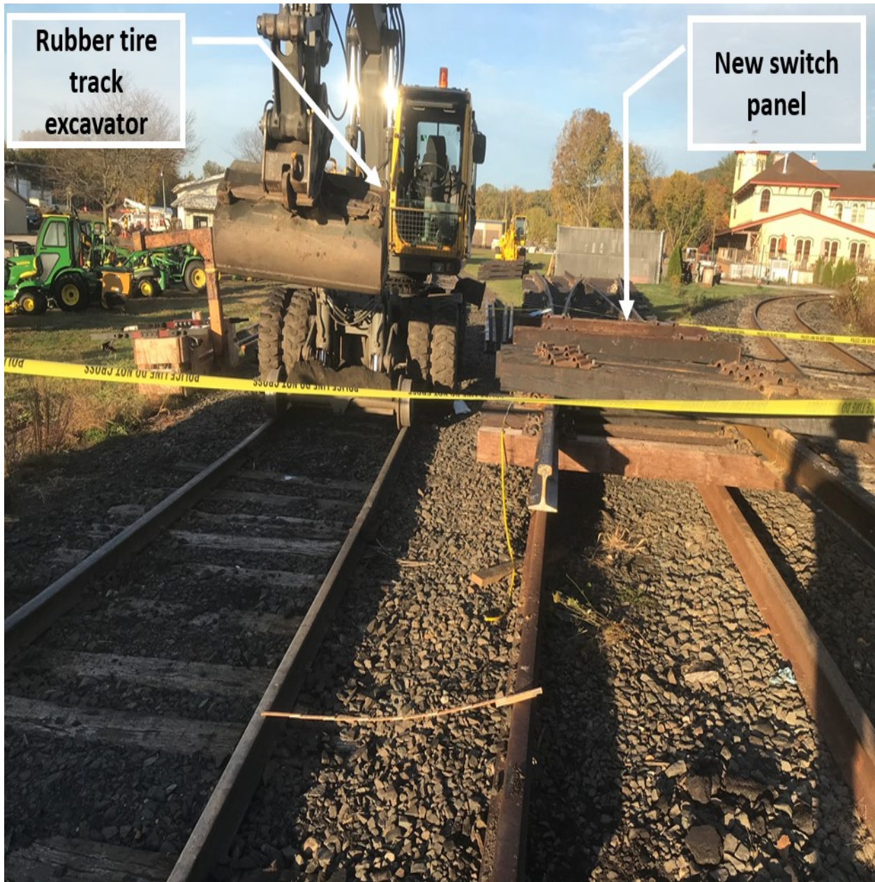
Figure 2- Excavator sitting on the tracks at the accident site.
