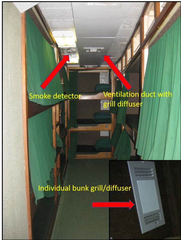
Figure 6. Port side of the Conception's bunk room looking aft, with inset of grill/diffuser (Source: Ryan, Inset: Landis).
