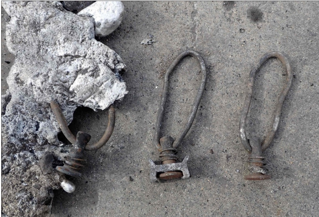
Photo 7: Deformed/Stretched Floor Tethering Rings
