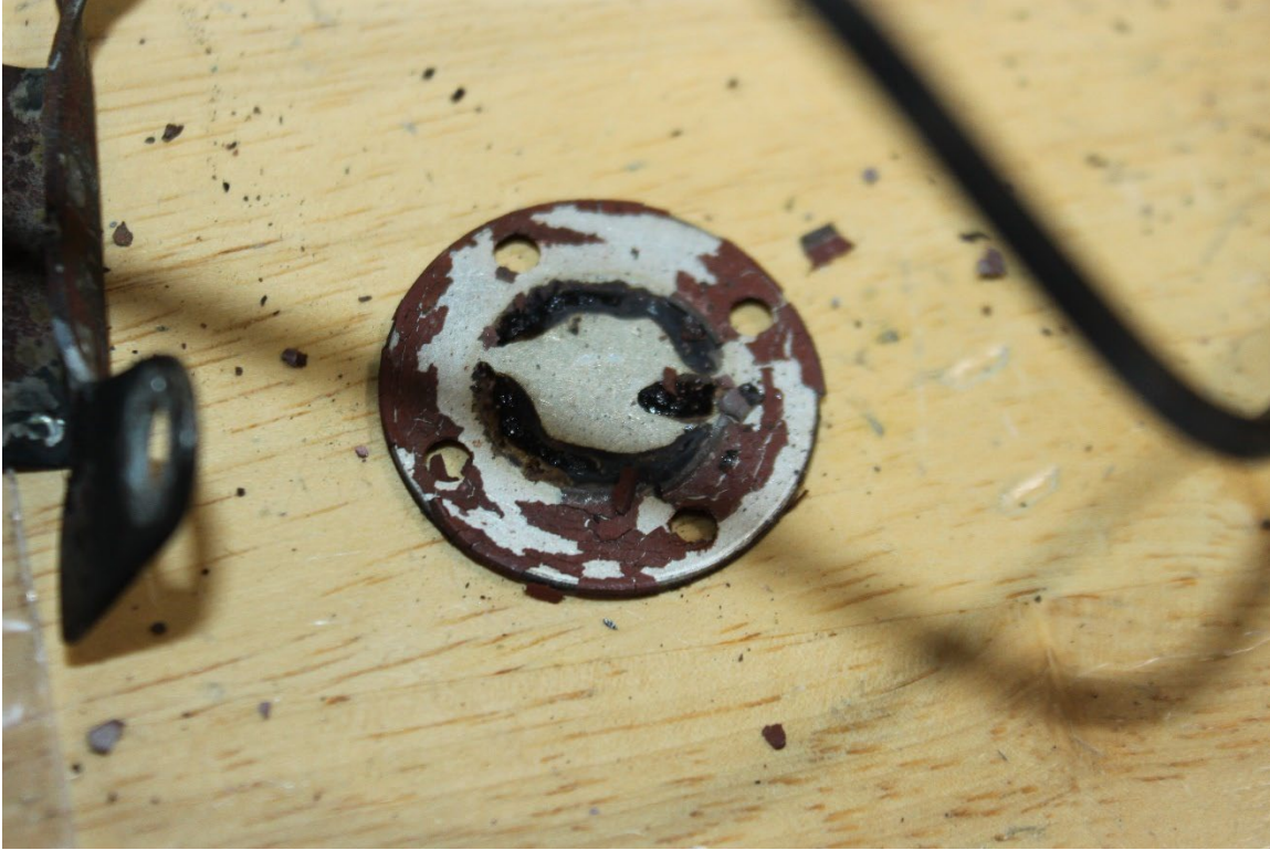
Figure 8: View of the Heat Damaged Gasket Following Removal Of the Bottom Cover of the Manifold Valve.
