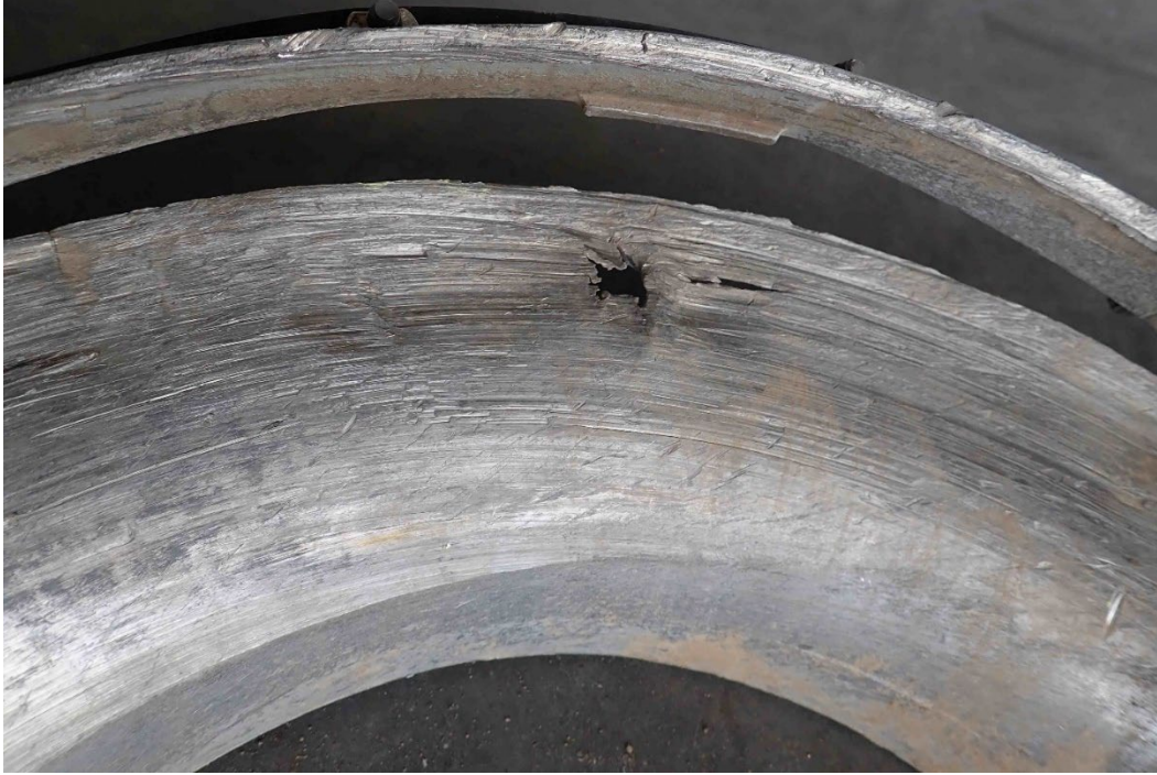
Photo 58 – Number 2 compressor shroud inner surface
