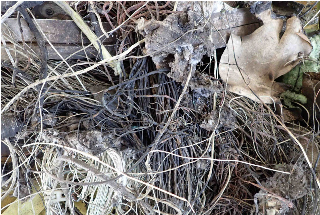
Photo 9 – Thermal damage to electrical loom
