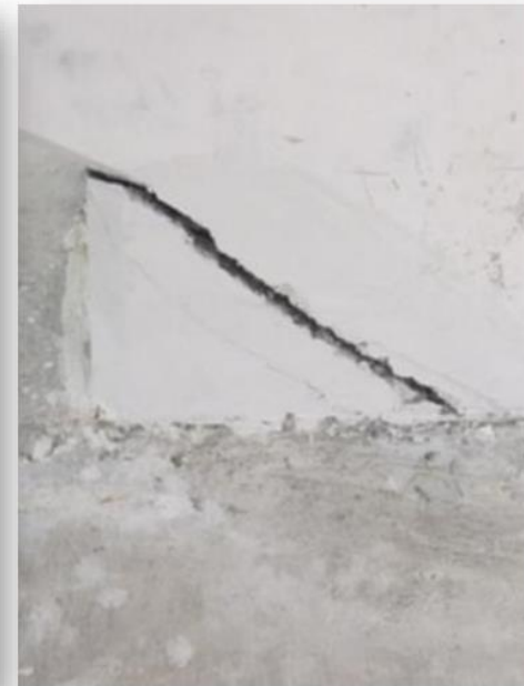
Same diagonal “wedge” crack 3 hours after the move. Photo taken by Molina at about 3 p.m. on March 10.
