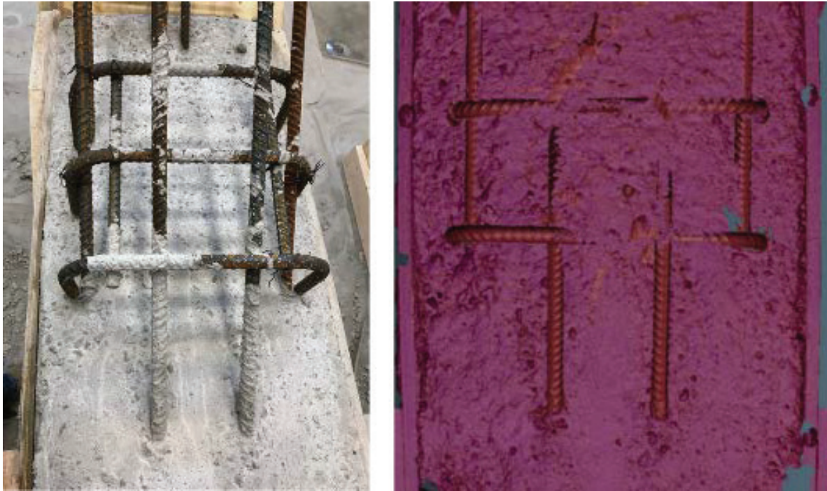
(a) As-placed (non-roughened) specimen construction joint (left) and laser scan of surface (right)
