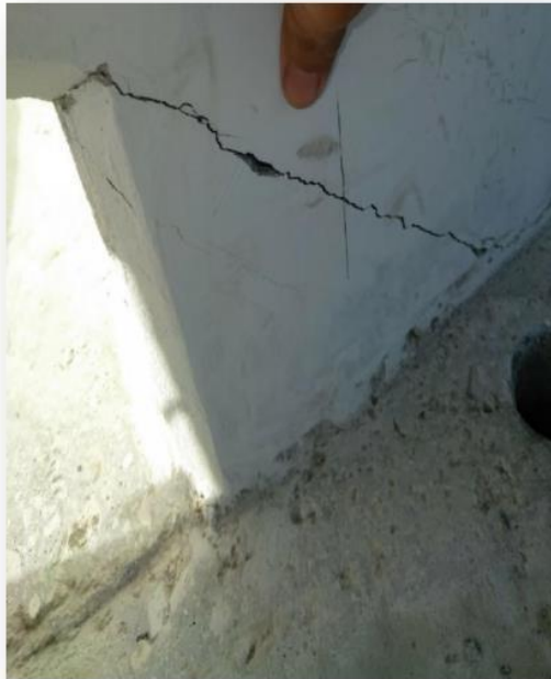
Diagonal “wedge” crack along the bottom of Diagonal 11 on the east face. Photo taken by BPA prior to the move on February 24, 2018.
