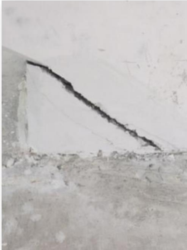
Diagonal “wedge” crack at base of Member 11 after the move on the east face. Photo taken by Corradino on March 10, 2018 at 3:07pm.
