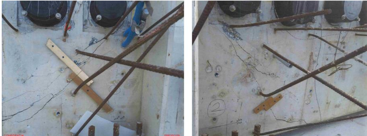
Figure 8.1. Wood blocks mounted across cracks on the north face of the north and diaphragm
