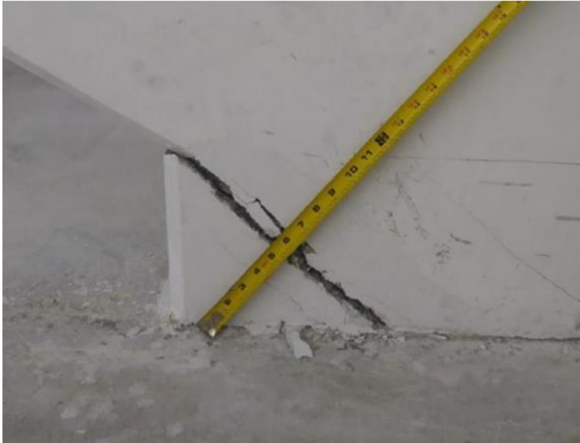
Diagonal “wedge” crack at base of Member 11 on the east face. Photo taken by MCM on March 12, 2018.
