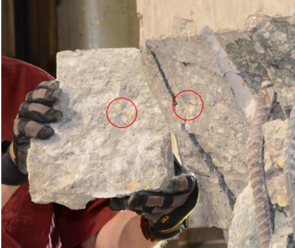
Figure 4.14. Construction joint interface of Specimen 5 (roughened, cracked) after failure. Circled areas show corresponding fractured aggregate on each side of interface.
