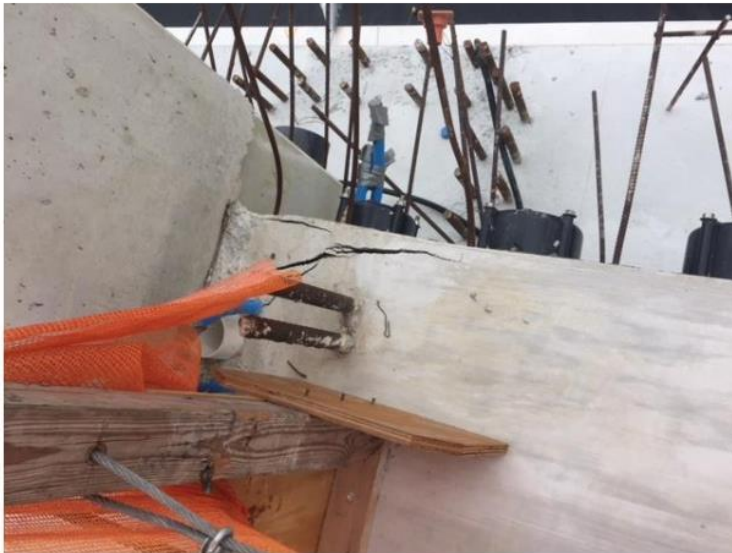
East side of Member 12. March 10 photo by Corradino showing same crack after move at 3:14 p.m.
