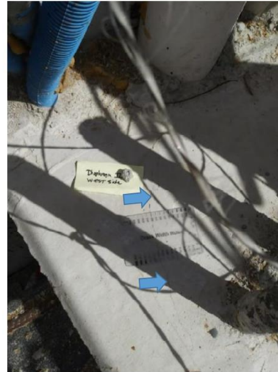
West side of Member 12. Photo 12 from BPA crack inspection report after formwork/scaffolding removal, February 28. Crack is indicated by blue arrows. Crack width ruler appears to indicate 0.014 inches.
