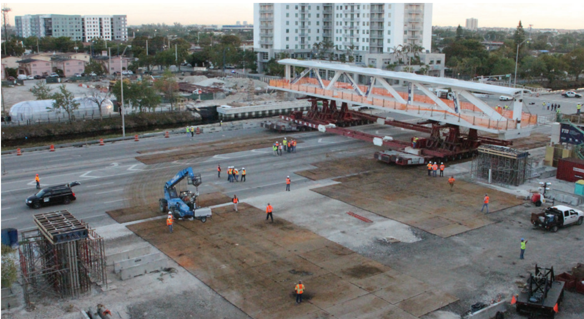
Precast main span truss move by transporters on March 10, 2018 from casting area to permanent piers. (Source: FIGG)
