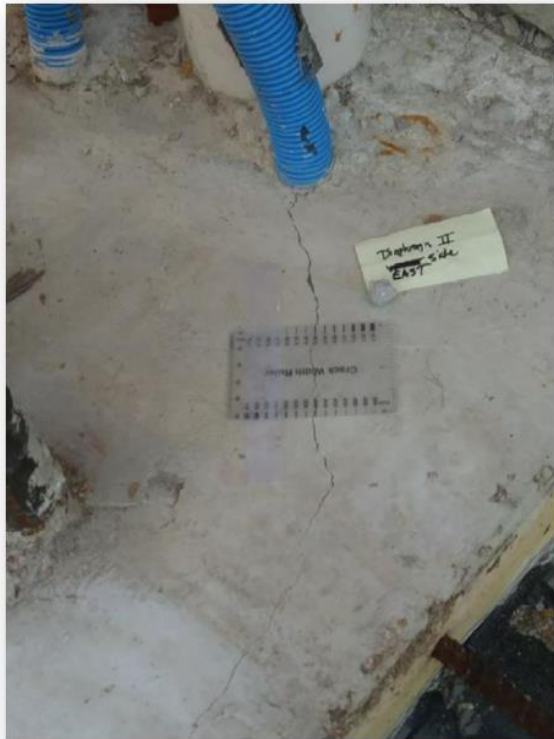
Photo 13 from BPA crack inspection after formwork/scaffolding removal. February 28.
