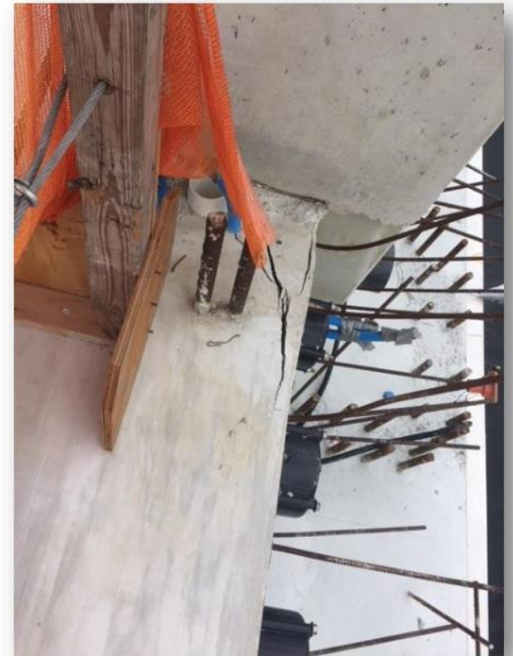
March 10 photo by Corradino showing same crack after move at 3:14 p.m.
