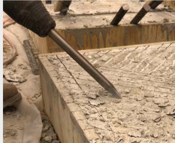
FIGURE 6-22 Electric chipping hammer and tool bit used to roughen specimen joint surface in accordance with FDOT Standard Specifications. (Source: WJE)
