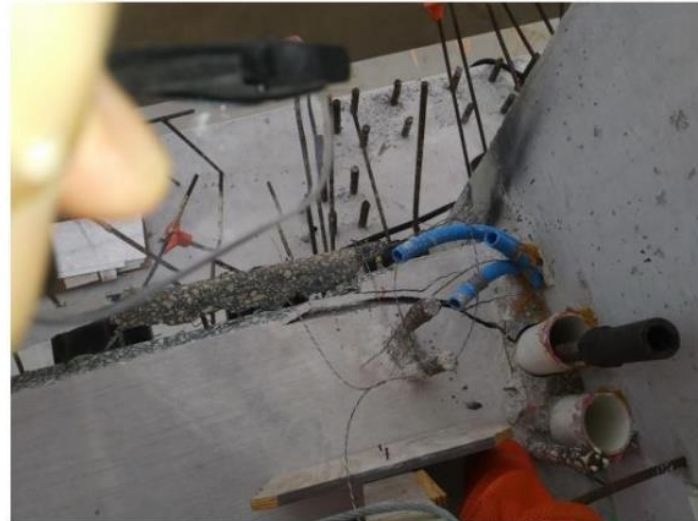
PHOTO 1: Diaphragm 2, Westside top view, crack
