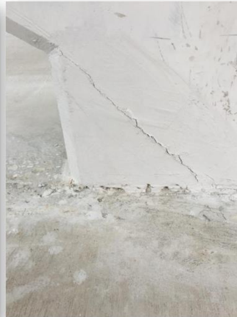
Same diagonal “wedge” crack shortly after the move. Photo taken by FIGG at about 12:30 p.m. on March 10.
