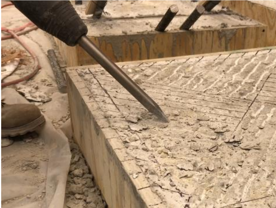
Figure 4.6. Roughening operation using an electric chipping hammer with amoil point (trial slab shown)
