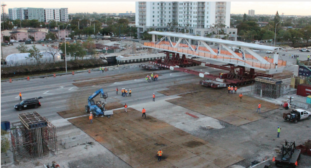
Precast main span truss move by transporters on March 10, 2018 from casting area to permanent piers. (Source: FIGG)
