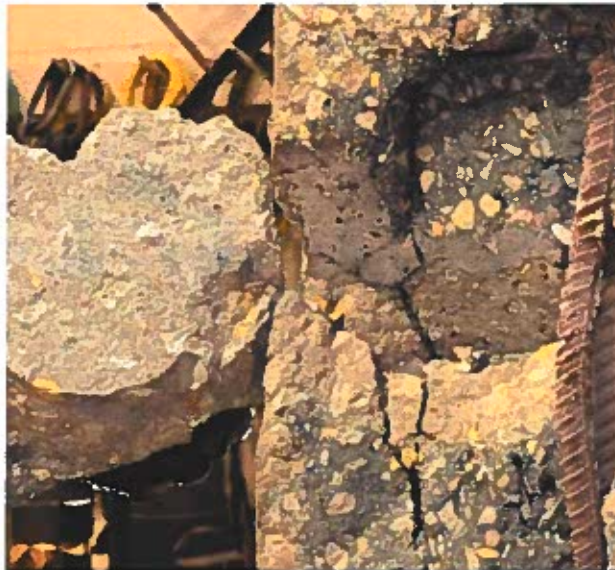
No Fractured Aggregate Non-roughened Joint Interface
