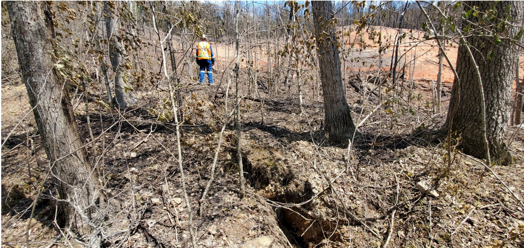
Photo C-5. Looking southeast (upslope) at lateral cracking on the northern flank of the landslide downslope of the TETLP ROW. Note tree roots in tension across the crack. This area is also where unburnt roots were observed, indicating additional movement following the FCI. BGC photo taken May 7, 2020.
