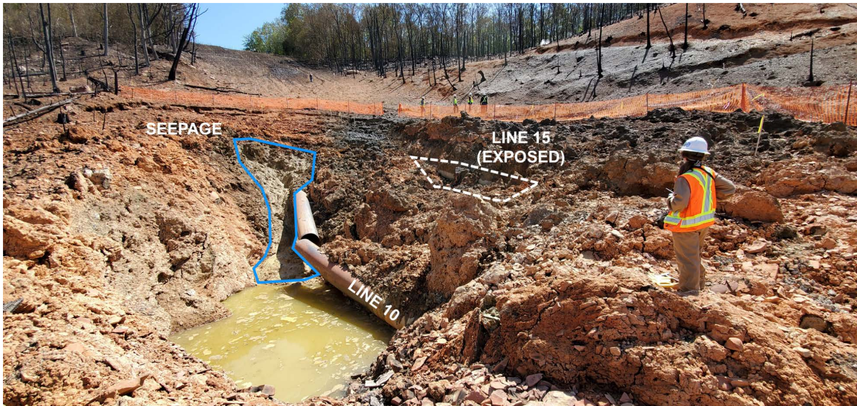
Photo C-2. Looking northeast (upslope) at the Line 10 blast crater. The failed girth weld is GW 11330. Seepage can be observed from the Line 10 trench backfill on the upslope side of the crater. Note the unstable material calving off the right (upslope) wall. Line 15 is within the upslope wall. BGC photo taken May 7, 2020.
