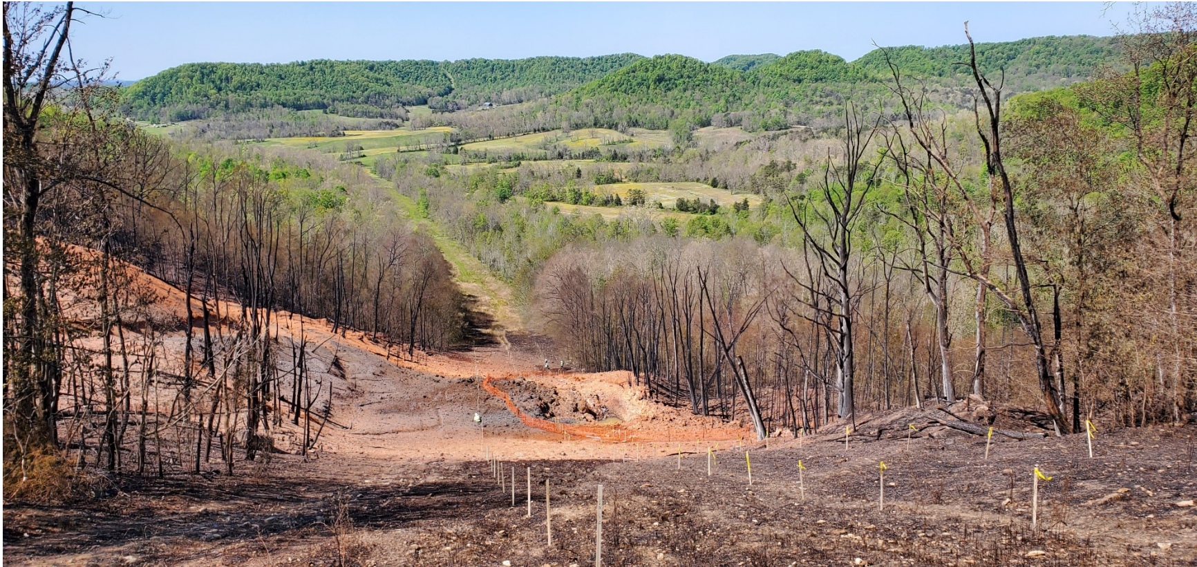
Photo C-1. Looking southwest at the FCI site. The blast crater from the FCI is within the orange safety fence in the middle portion of the photo. BGC photo taken May 7, 2020.
