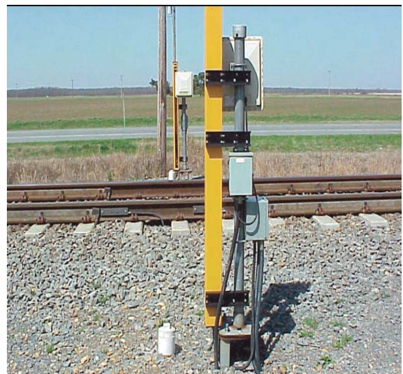
Figure 11: A Typical Low Air-Hose
