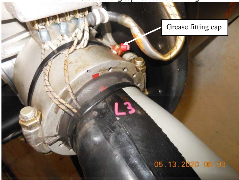
Photo #4 – Grease fitting cap not secure on fitting
