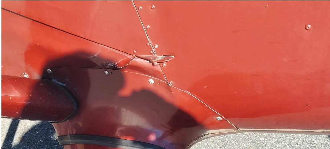
Photograph 3 - Fuselage Damage (Courtesy of Pilot)
