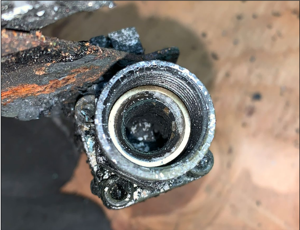
Photo 7: View of the cross feed valve as found mostly closed and seized, but with a partial opening.
