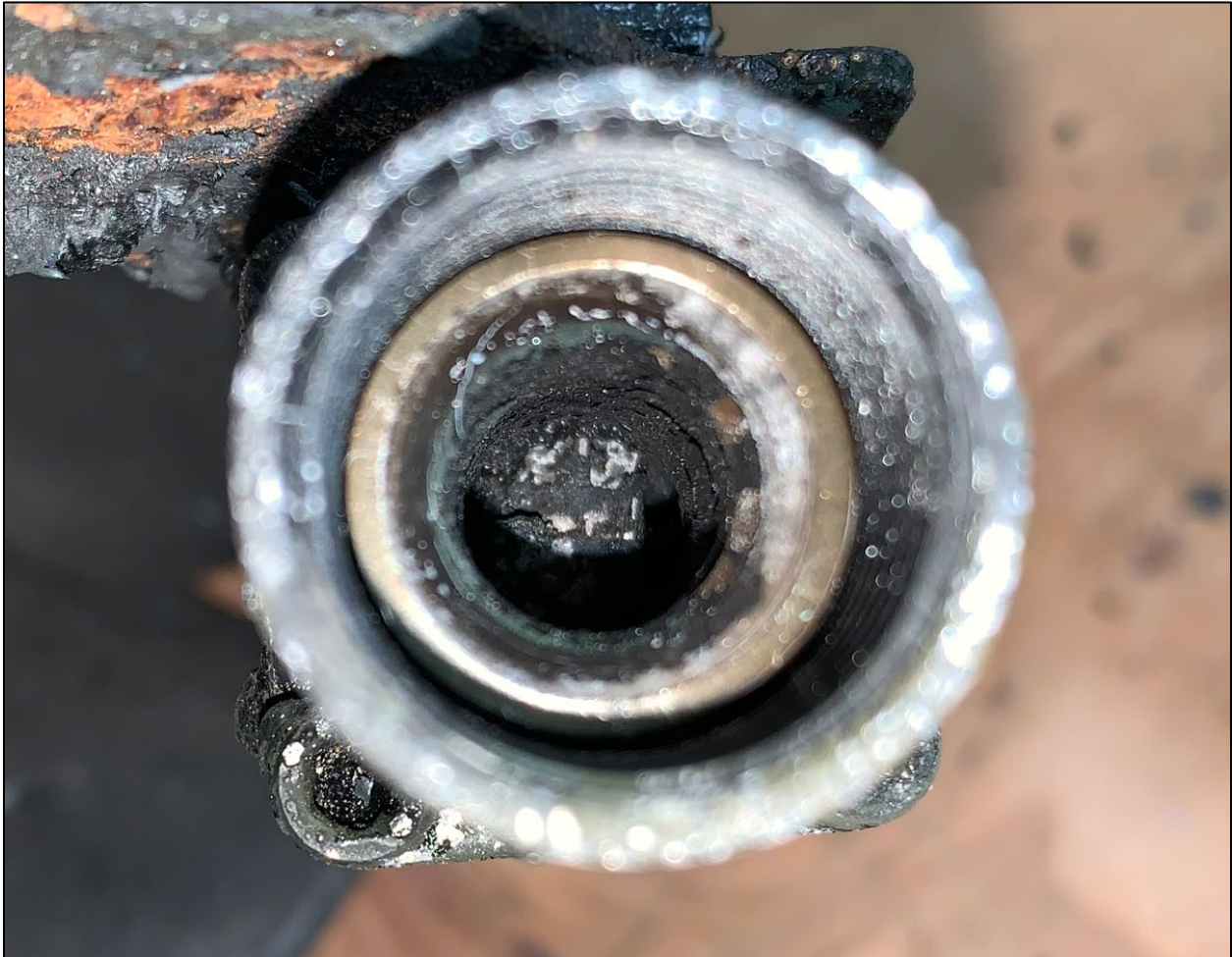
Photo 8: Additional view of the cross feed valve as found mostly closed and seized, but with a partial opening.
