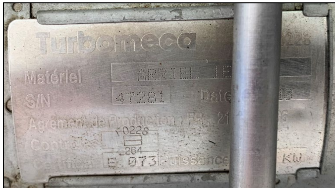
Photo 1: Left No. 1 Engine Data Plate.
