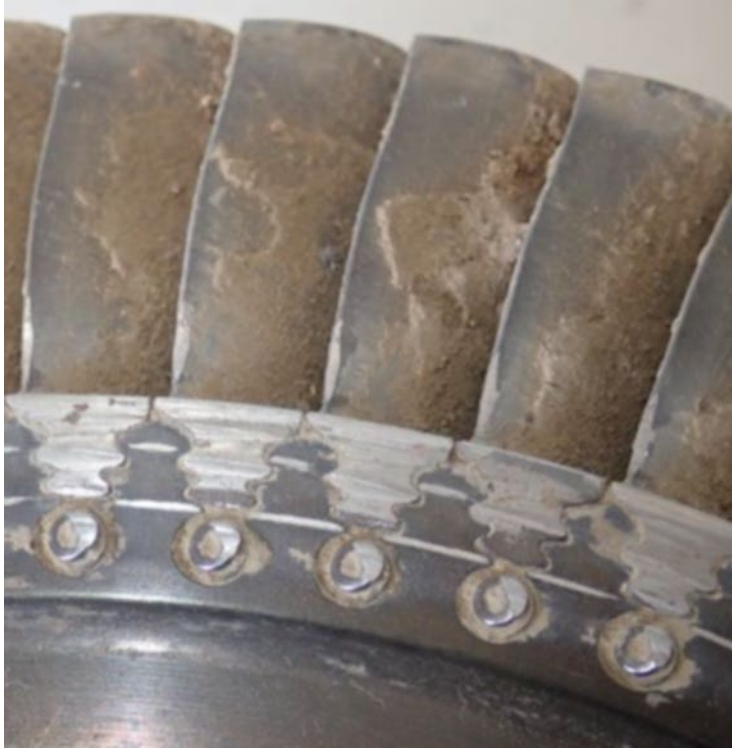
Figure 5. High turbine downstream face showing circumferential scoring along the blade retention rivets, fir tree root area, and blade platform and trailing edges
