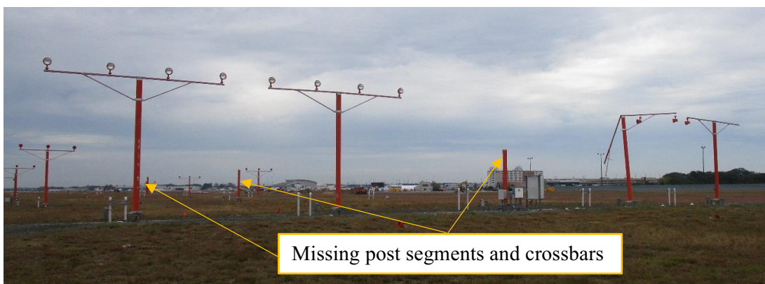
Figure 36 Damaged approach lighting
