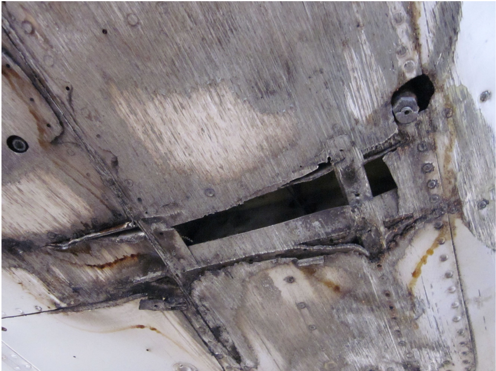
Photo 2 – Structural damage to the underbelly (Courtesy of FAA)
