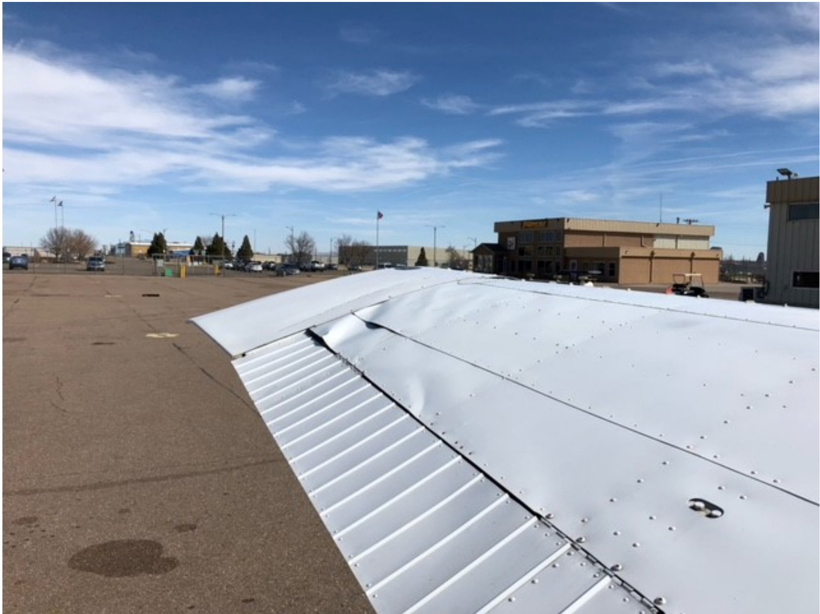
Photo 1 – Left Wing Damage (Courtesy of the owner)
