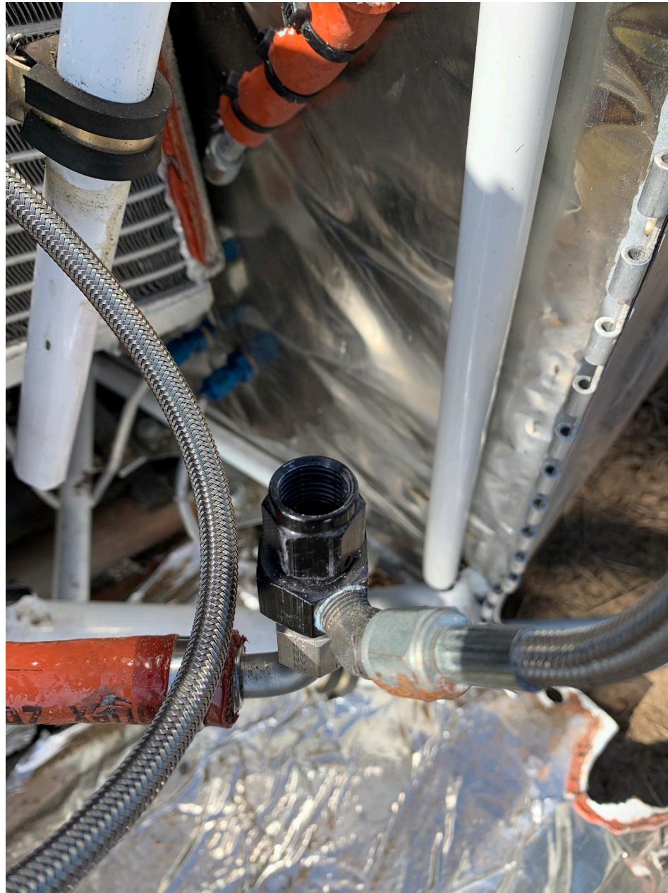
Photo 4 - View of Disconnected Adapter Fitting (FAA)
