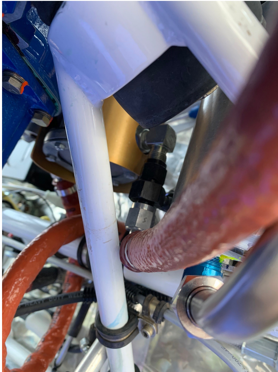
Photo 3 - View of Adapter Fitting as Installed (Owner)
