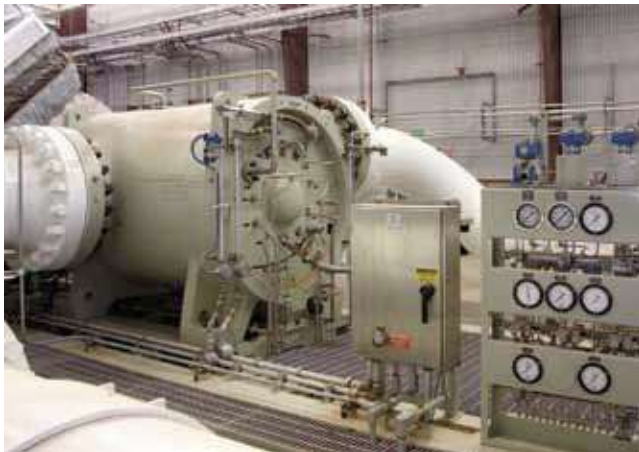
C65 Gas Compressor
