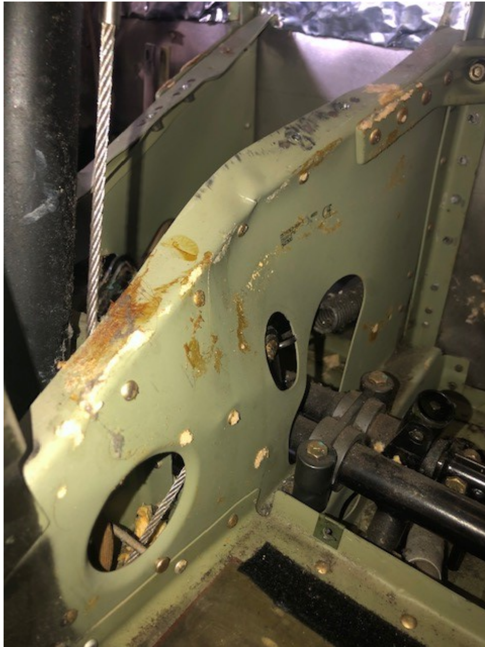
Photo 1 – View of bulkhead assembly damage (photo courtesy of the operator)
