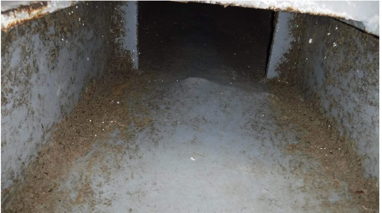
Photo 8 – Tainter Gate #7 - Deformation in Skin Plate (view on downstream side of skin plate between vertical ribs)
