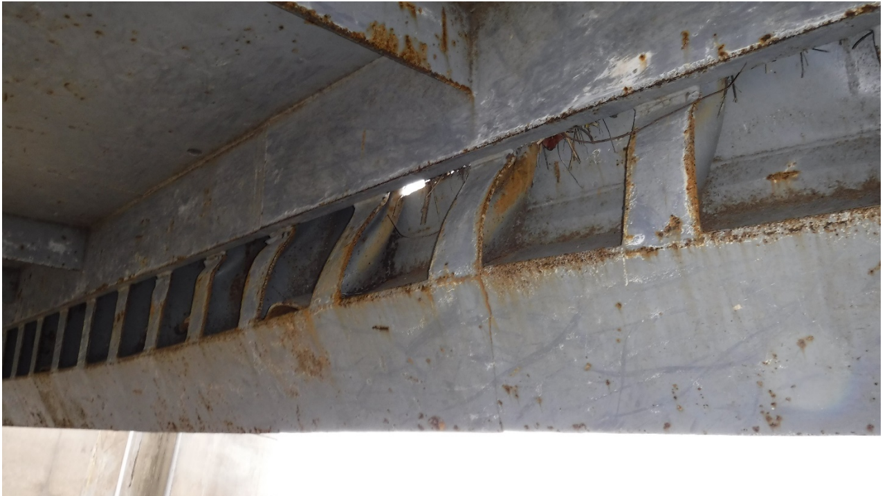
Photo 4 – Tainter Gate #5 – Deformed Vertical Ribs
