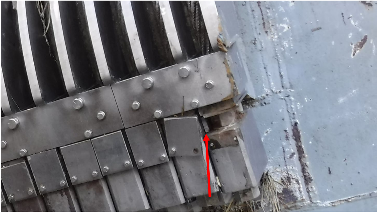
Photo 2 – Tainter Gate #4 - Zoomed in View of Fractured Nut and Washer Shim Plate on Inboard Cable Socket (Arrow indicates remaining portion of shim plate)
