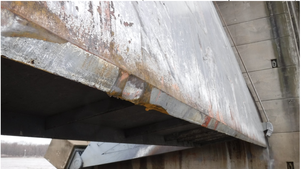
Photo 9 – Tainter Gate #7 – Gouge in Bottom Edge of Skin Plate
