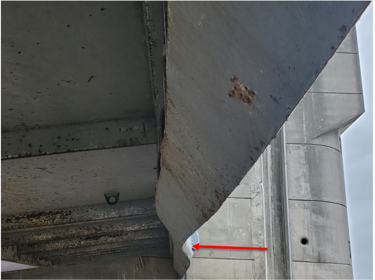
Photo 6 – Tainter Gate #5 – Approximate 6” Deformation in Bottom Portion of Skin Plate
