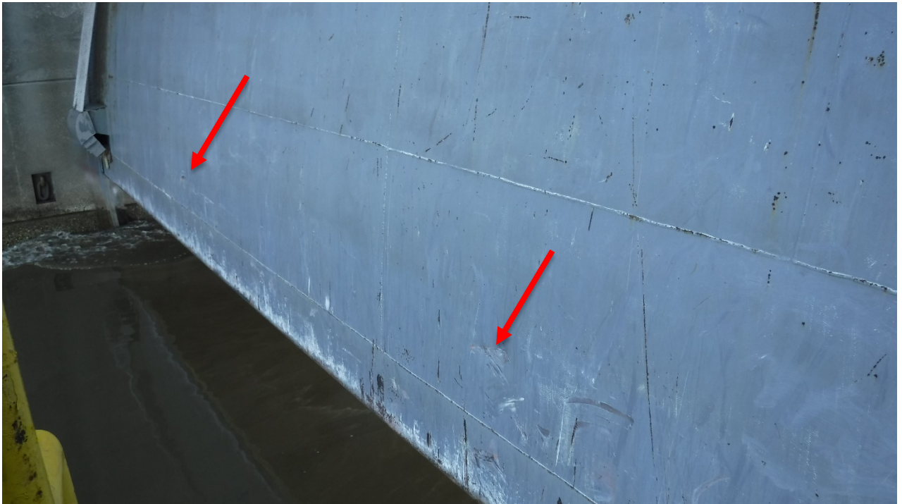
Photo 7 – Tainter Gate #7 – Deformations in Skin Plate
