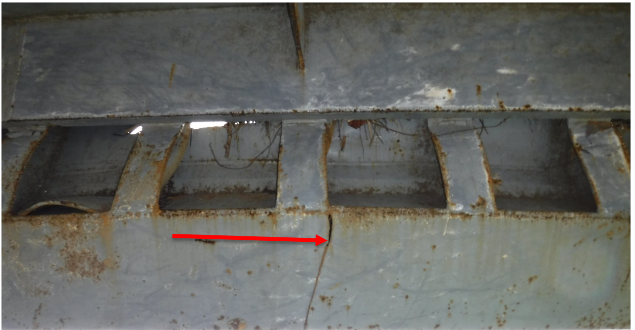
Photo 5 – Tainter Gate #5 – Fracture of 1” Steel Plate
