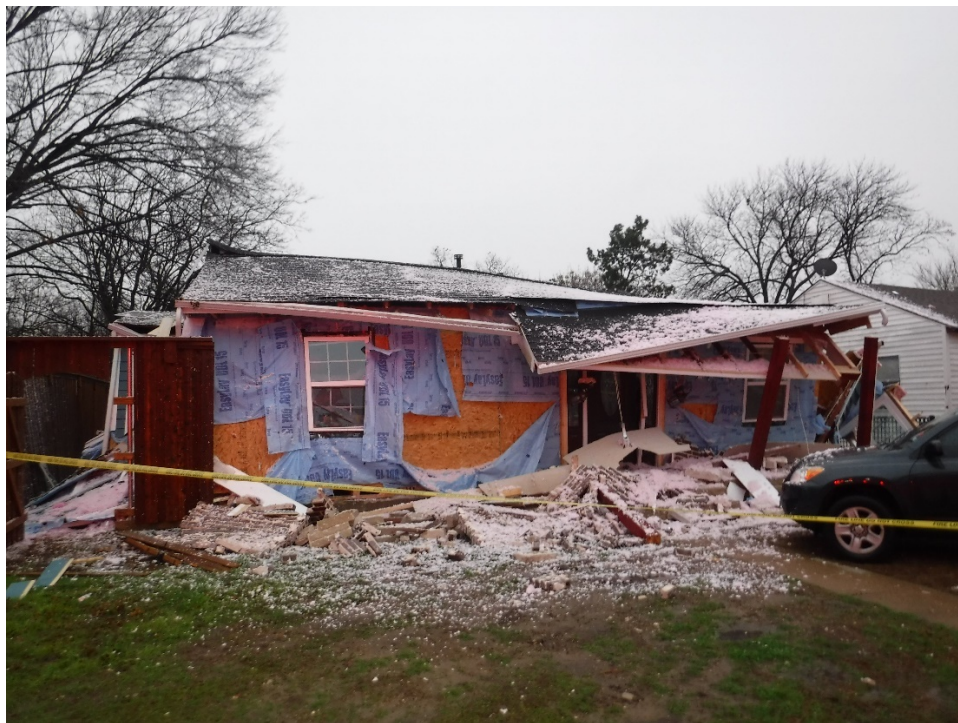
Figure 1: House 3534 Espanola Drive after the explosion on February 23, 2018
