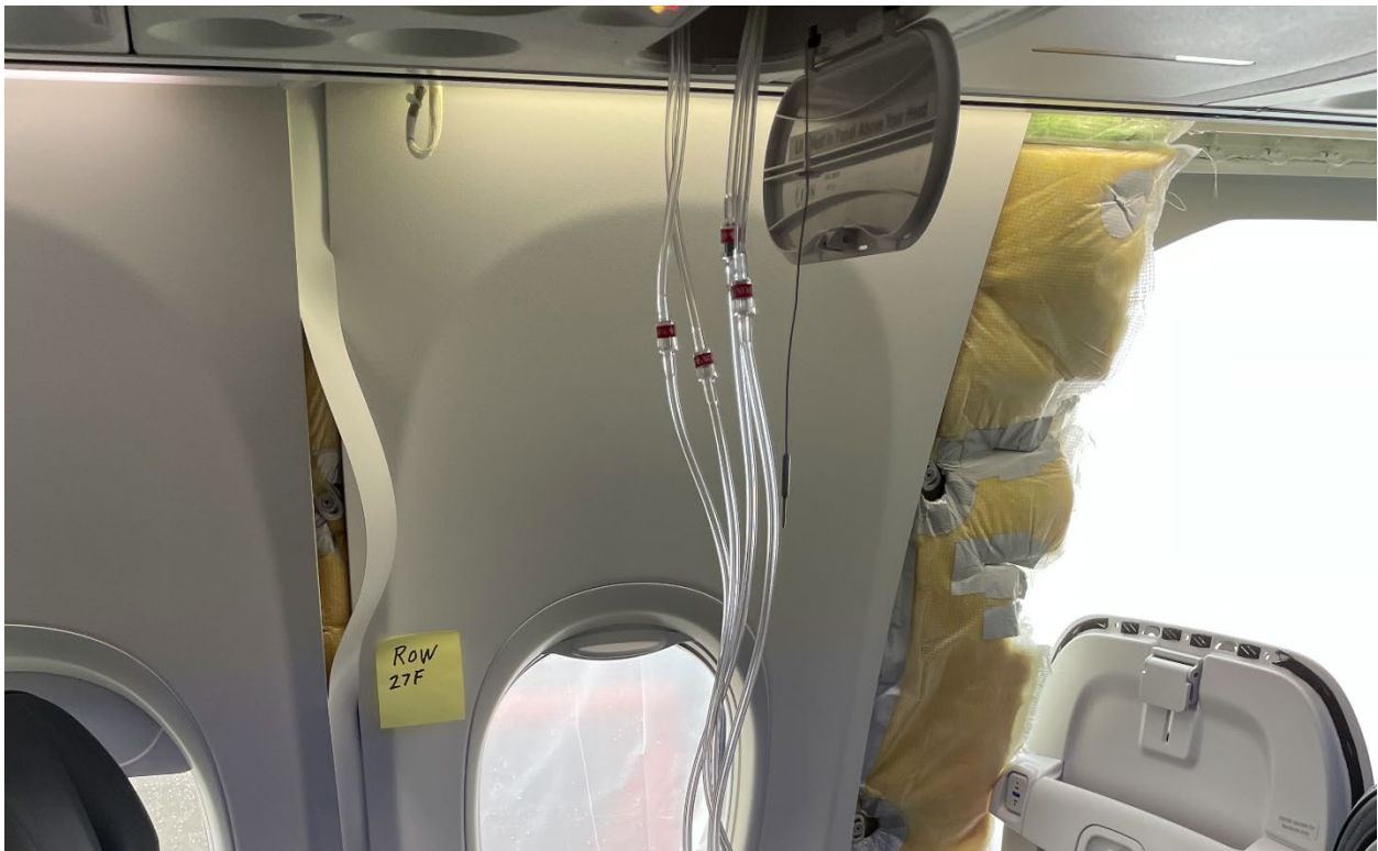
Figure 15. Sidewall trim strip buckled at row 27ABC.
