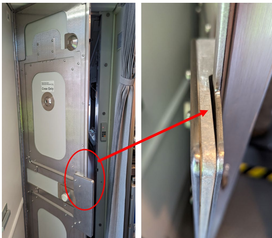
Figure 34. Area of deformation to the door latch security plate of the flight deck door.
