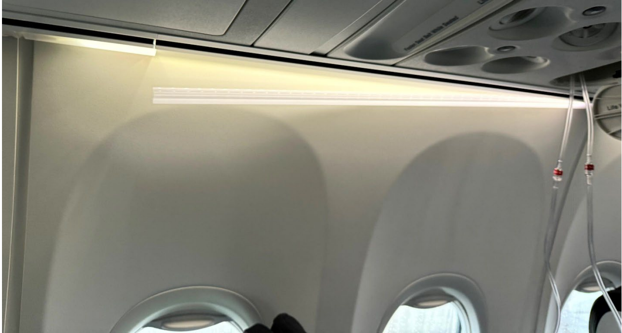
Figure 16. Loose sidewall cove light at 30-31ABC.
