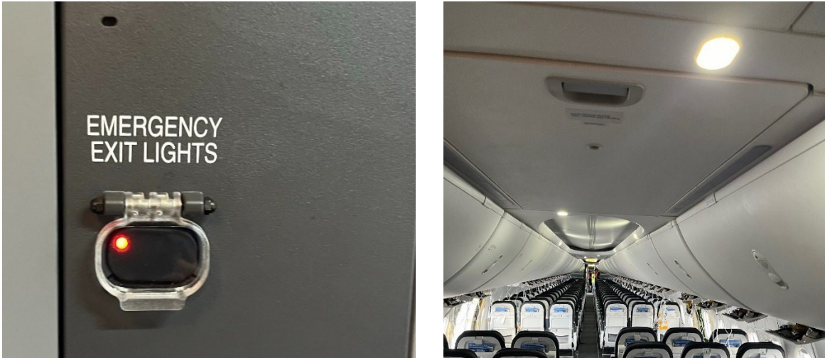
Figure 24. Emergency lighting activation switch at the door L2 F/A location and illuminated overhead light fixtures in the cabin.
