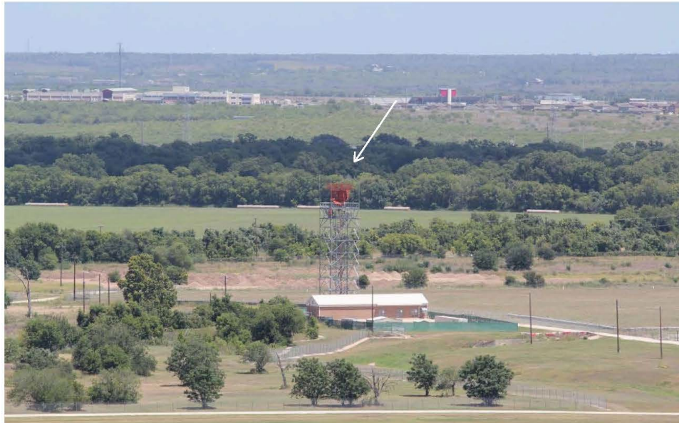
#13 1 E – ASR-9 Radar Antenna (Day/Night)
