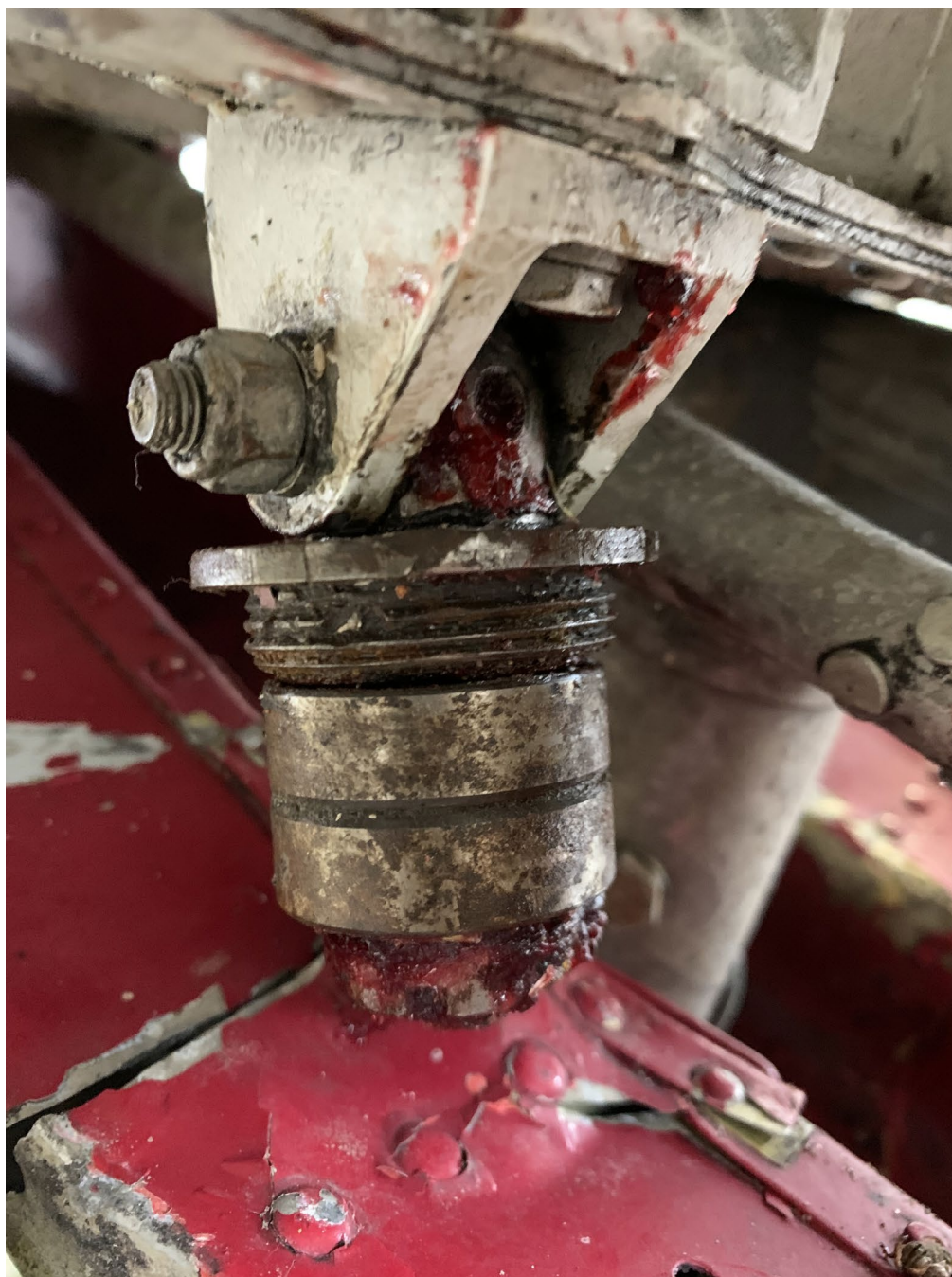
Figure 6. Horizontal stabilizer trim actuator top eye end and bearing assembly as found attached to the horizontal stabilizer mounting bracket (NTSB photo)
