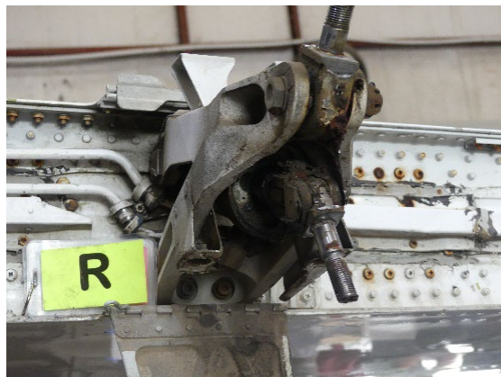
Figure 38. The right-hand hydraulic boost cylinder, as installed.
