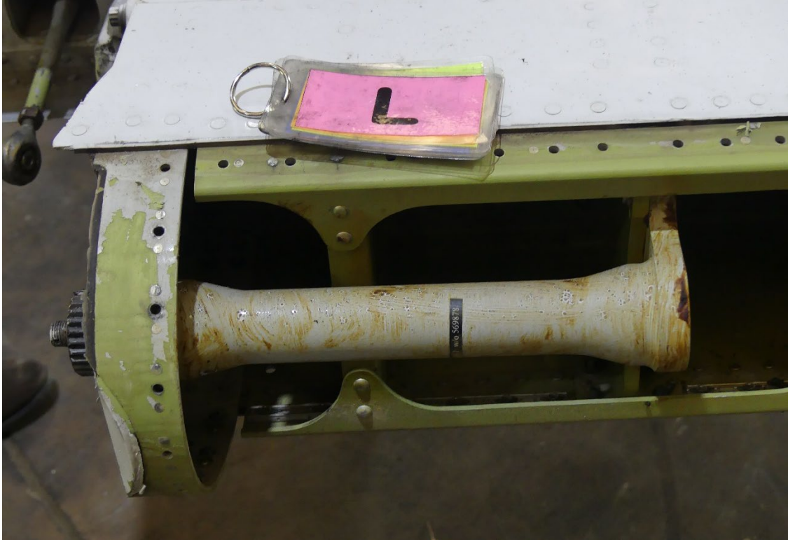
Figure 41. The left elevator torsion bar, as installed.
