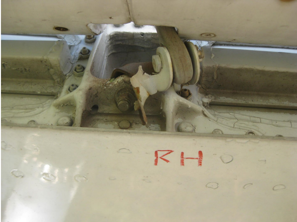
Figure 27. Right-hand elevator inboard geared tab attachment linkage, looking forward into the horizontal stabilizer, viewed from underneath the right elevator.
