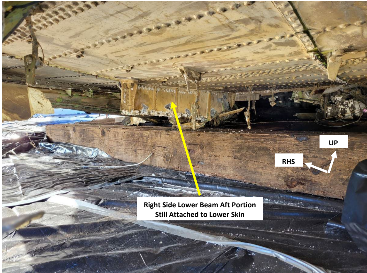
Figure 57. WCS Lower Skin right Lower External Beam attach point damage (Boeing photo)
