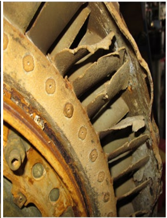
Figure 19 Detail of Figure 18 showing C7 blade LE damage and full-length C8 blades
