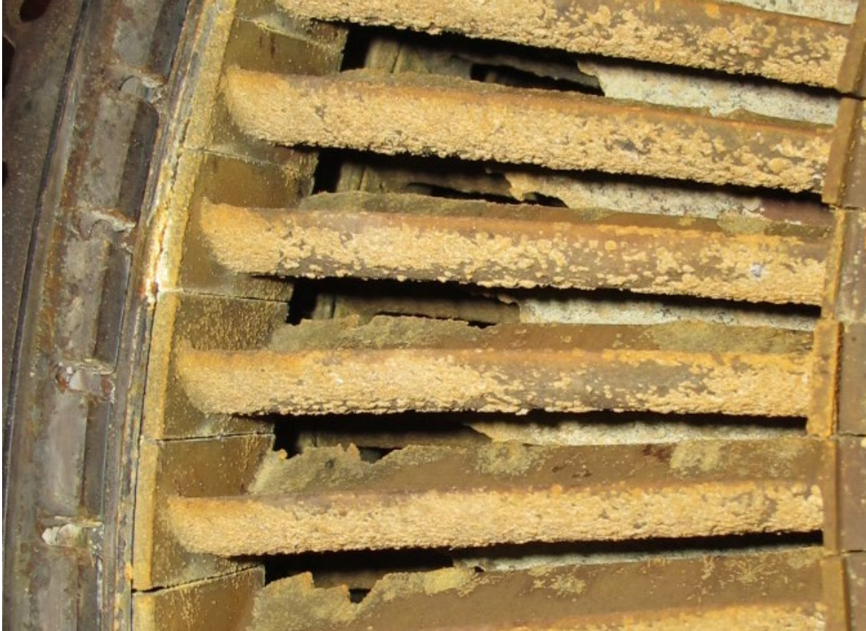
Figure 41 Detail view of No. 2 engine T2 blade outer span damage
