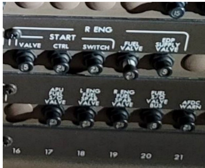
Figure 21 - Right EDP Supply Valve circuit breaker on incident airplane
