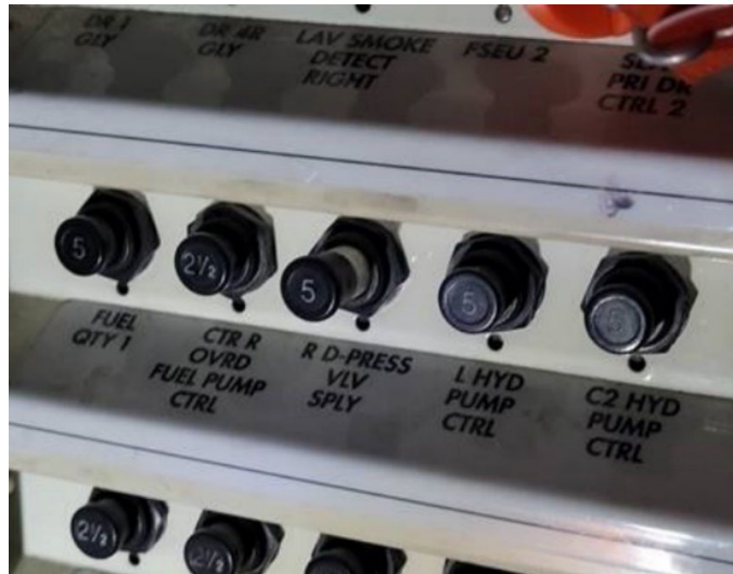
Figure 26 - Depressurization solenoid valve circuit breaker on incident airplane
