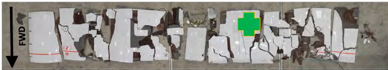
Figure 90: Fan cowl thermography results.
