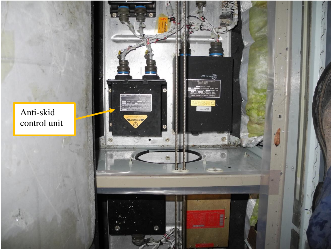
Figure 36 Antiskid control unit (left side of image)
