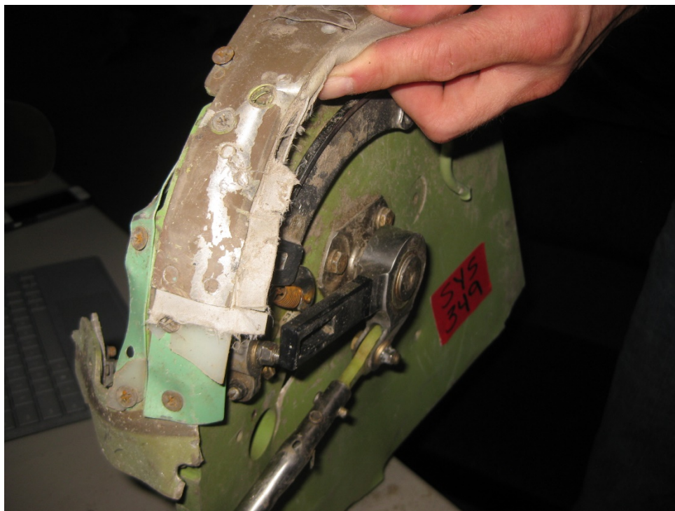
Figure 15 - Speed Brake Rail with finger pointing to the compressed area of the outer frame.
