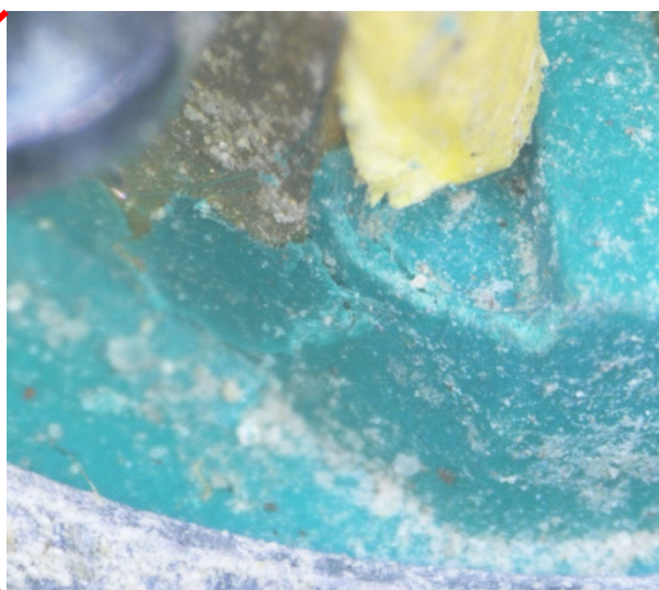
Figure 30 – Cracking noted in switch base
