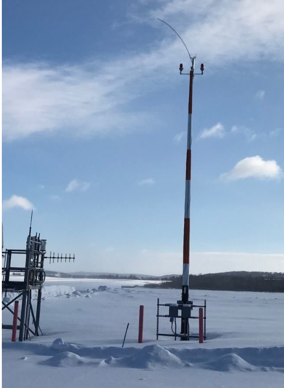
Figure 5 AWOS wind sensor tower (source: NTSB)
