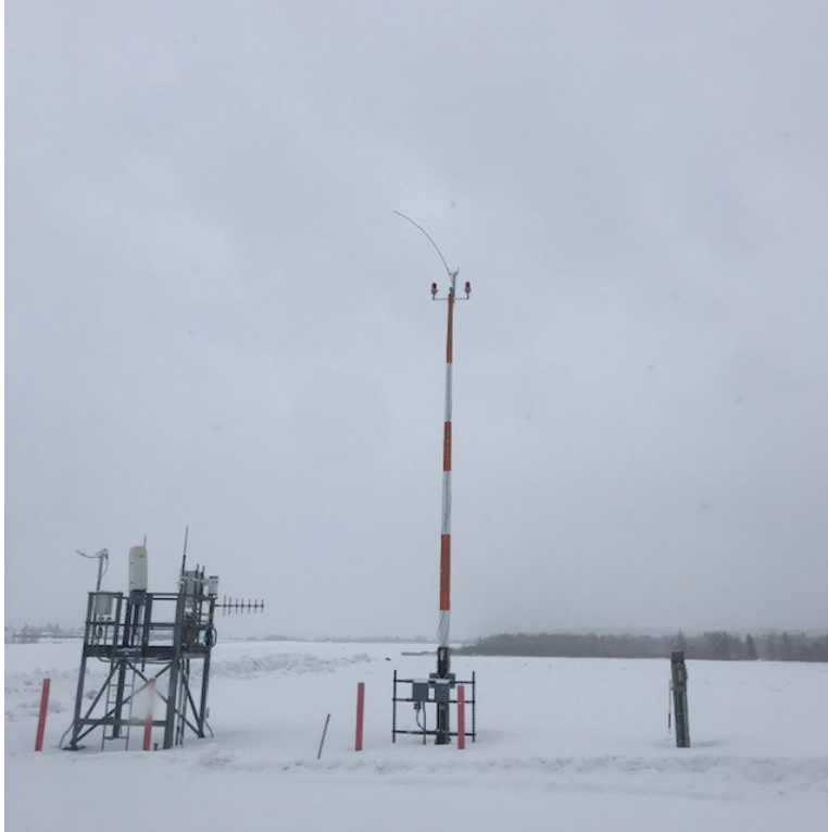
Photo 8. Bent lightning arrester on AWOS wind sensor pole (courtesy PQI).
