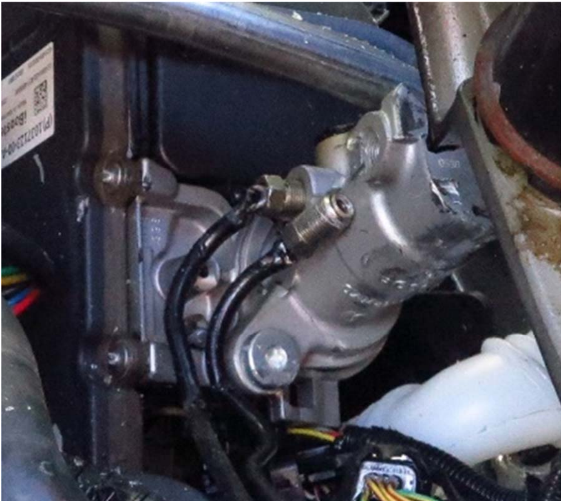
Vehicle Photo 4: This is a view of the damaged brake master cylinder for the passenger vehicle.
