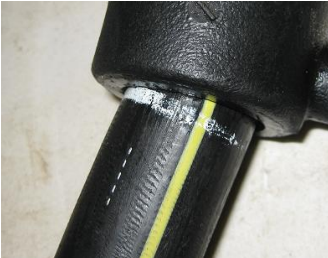
Figure 8 –Picture of insufficiently scraped 1" PE pipe
