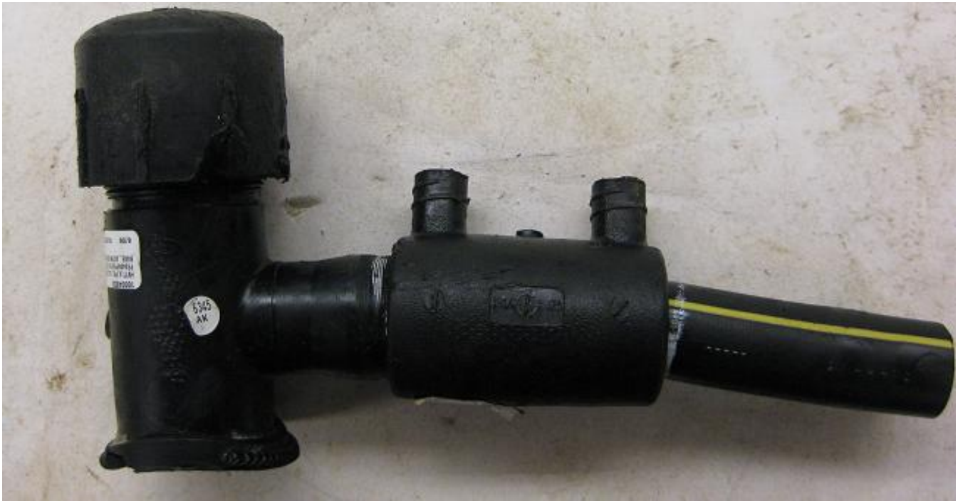
Figure 7 –Picture of misaligned pipe and reducer on tapping tee
